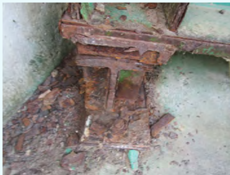
Heavy section loss of rocker bottom
