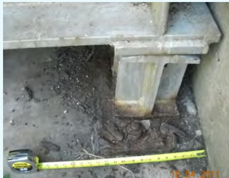
Poor alignment w/ masonry PL
