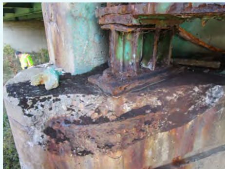
Loss of bearing on masonry of sub unit
