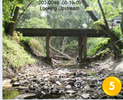
Trees and brush restrict channel.
