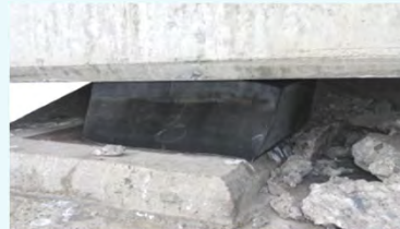
Excessive shear deformation / location
