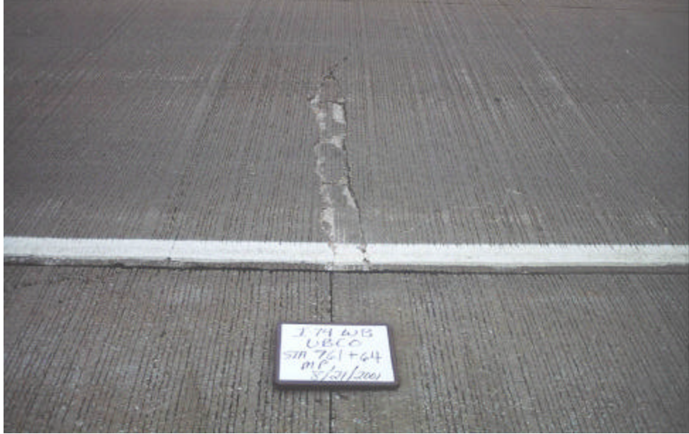
Figure 1. Early Stage of Punchout in Unbonded Concrete Overlay in 2001.
