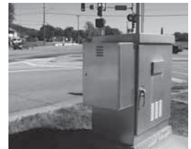
UPS unit and batteries in a piggyback cabinet; the design is suitable for retrofitting a signal cabinet for UPS equipment.
