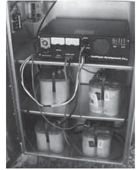
Installation of UPS in a separate, attached cabinet; the UPS unit is on the top shelf, and the batteries are on the middle and bottom shelves.
