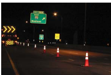
This photograph shows a three-lane, one-way roadway at night. Traffic cones are placed on the lane line closing the left lane. The cones are marked with two retroreflective white bands. A work vehicle with an Arrow Panel and Truck Mounted Attenuator is positioned in the closed lane.
