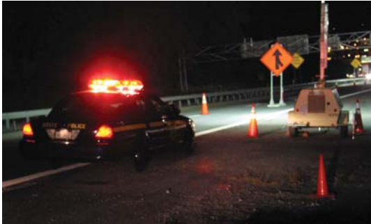
This photograph shows a police patrol vehicle stationed near a night work site. The rooftop warning lights are in operation, and the police markings on the rear of the vehicle are visible.
