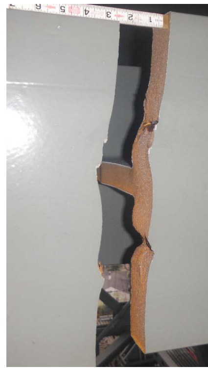
Figure 8 Close-up of north flange fracture face. (HNTB)
