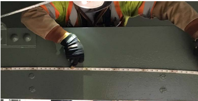
Figure 9 Tack-welded rivet shanks, member U19-19', near PP20 (HNTB)
