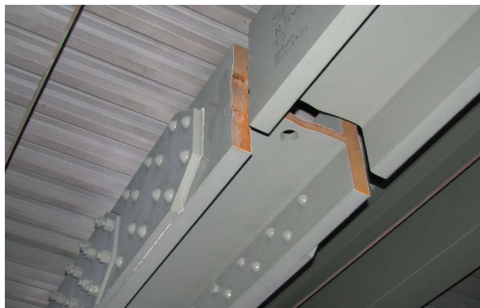
Figure 3 Fracture of U19-19', North Truss, Looking South and East at Panel Point 19', prior to any material sampling. (HNTB)
