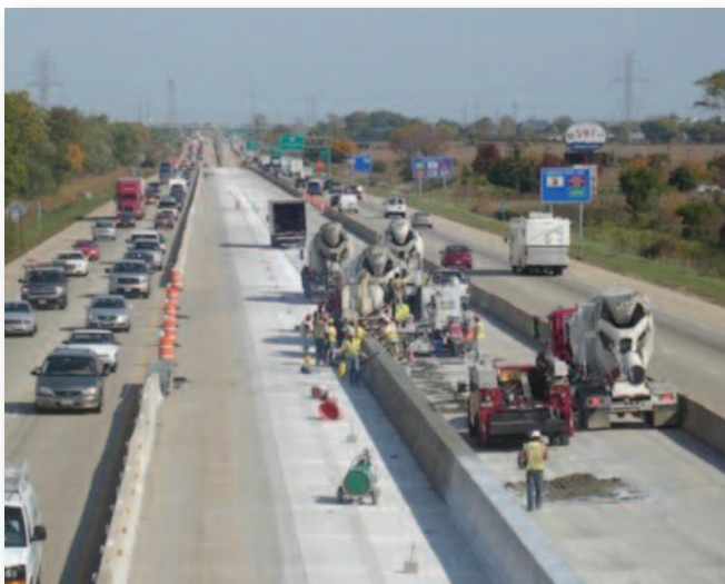
I-80 from US 30 to US 45 Work primarily consists of adding a median barrier wall and inside shoulders along I-80
