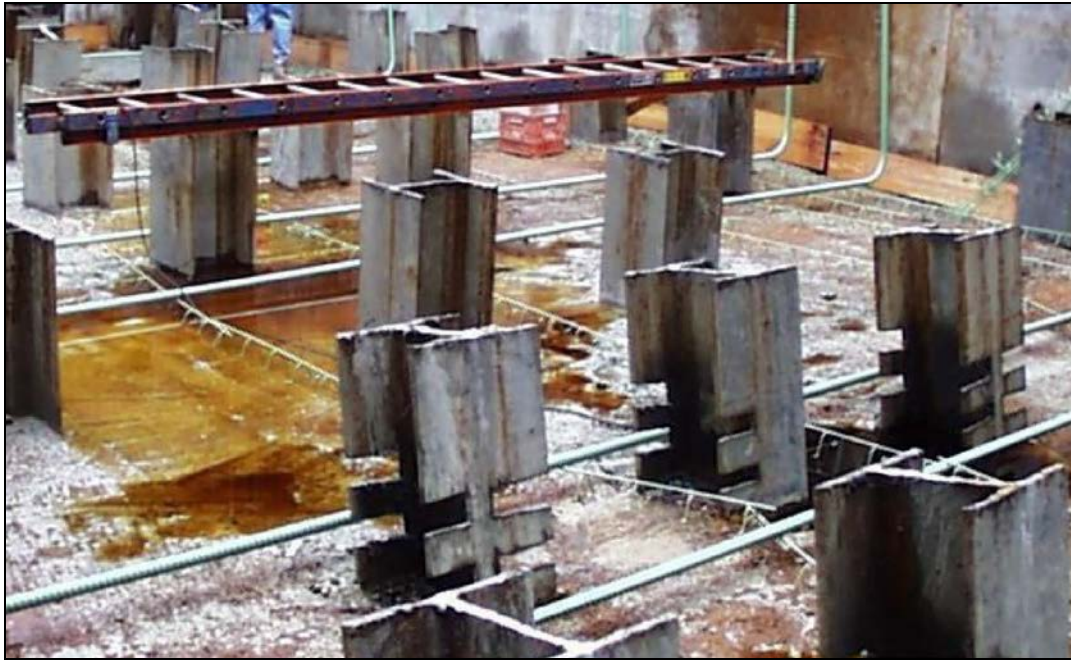
Example of Unacceptable Notches Cut into Piles
