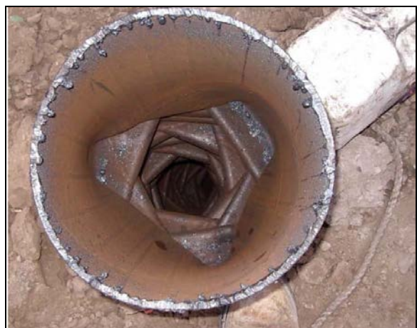
Damaged Metal Shell Pile
