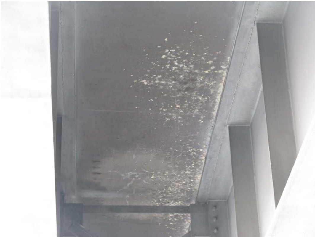
Photo 4 - Typical discolored concrete and pop off in Span 2, looking east
