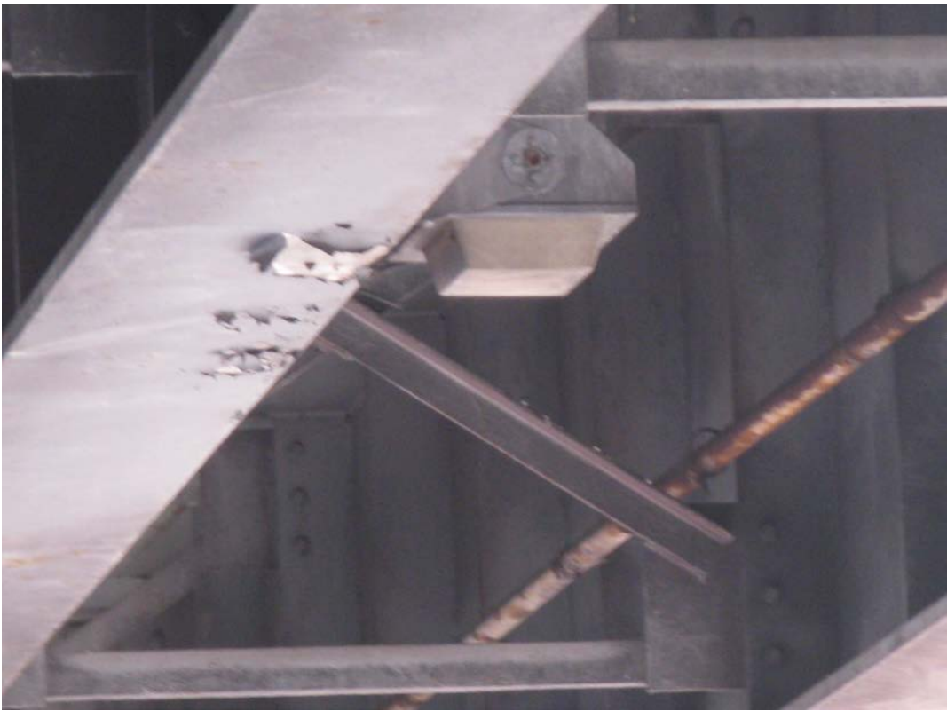
Photo 16 – Paint peel on Beam 9 in Span 2, looking east
