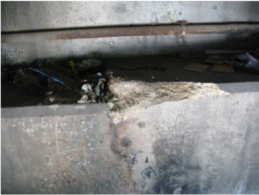
Photo 26 - Spall on West Abutment seat in bay 2 from north, looking east
