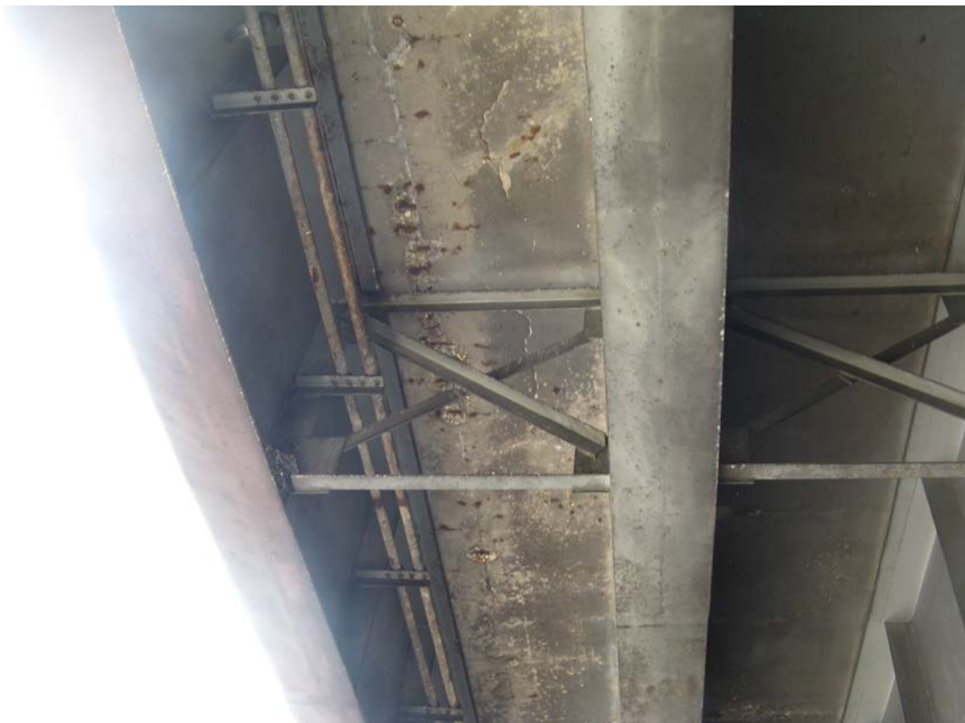
Photo 2 - Spalls on underside of deck in Span 2 between Beams 9-10 from north, east end, looking west
