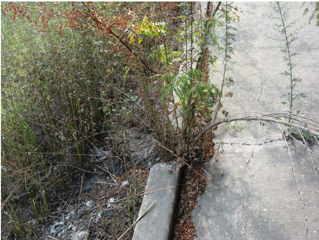
Photo 34 - Broken section of west slopewall curb with vegetation growing in it, approx half way up, looking west
