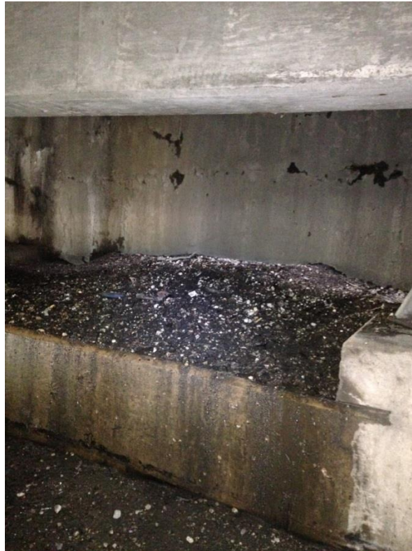
Photo 39: West abutment between girders 3 & 4 showing large deposit of sediment from the top of deck.
