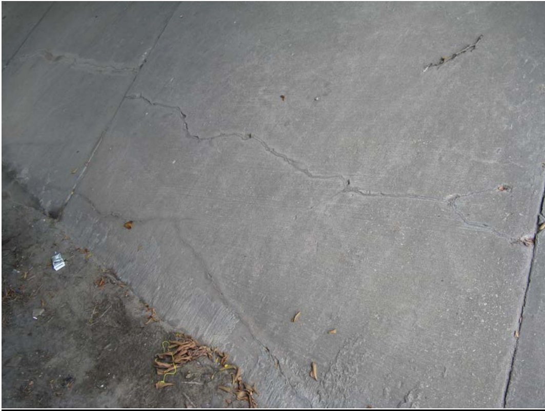
Photo 39 – Cracks in north end of west sloped wall, looking southwest
