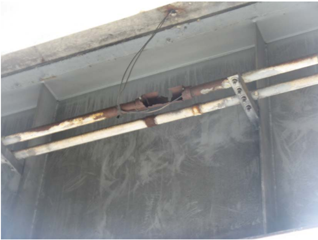
Photo 21 - Broken conduit in Span 2 along south fascia beam, 6' from West Pier, looking southeast
