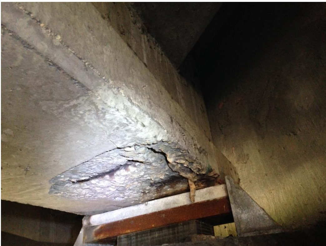
Photo 12: Underside of girder 6 over west abutment showing spalling with exposed and corroded reinforcement.
