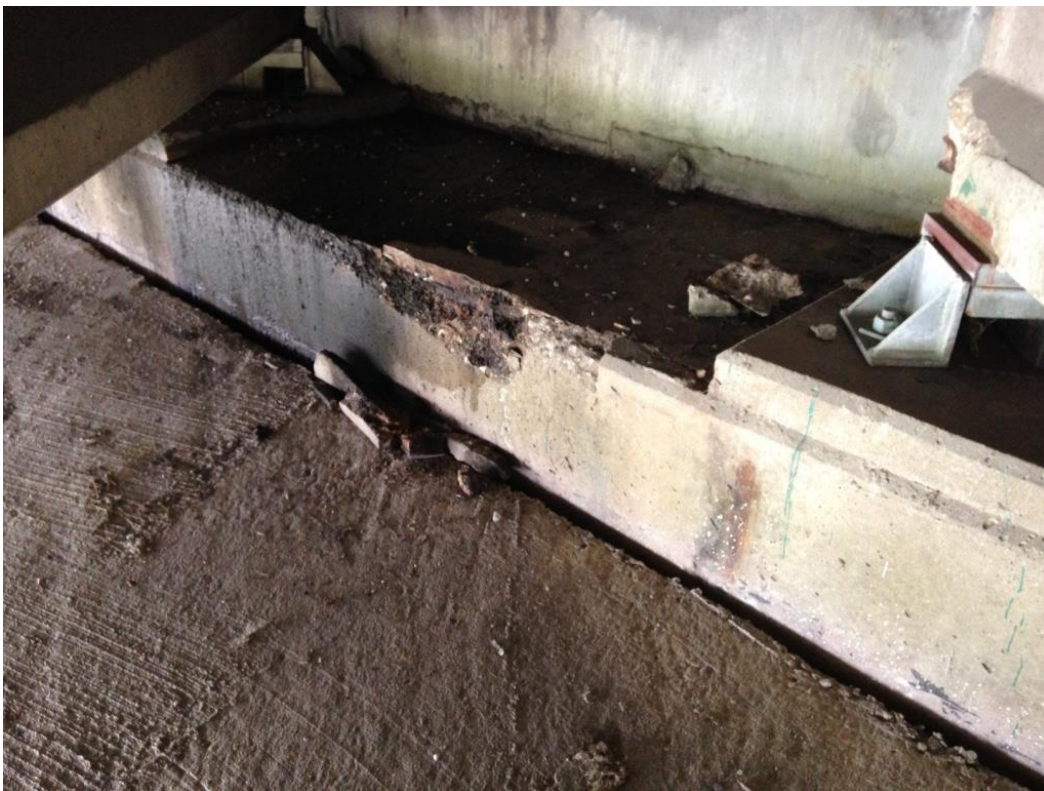
Photo 36: West abutment between 19 & 20 showing spalling with exposed and corroded reinforcement on abutment seat.
