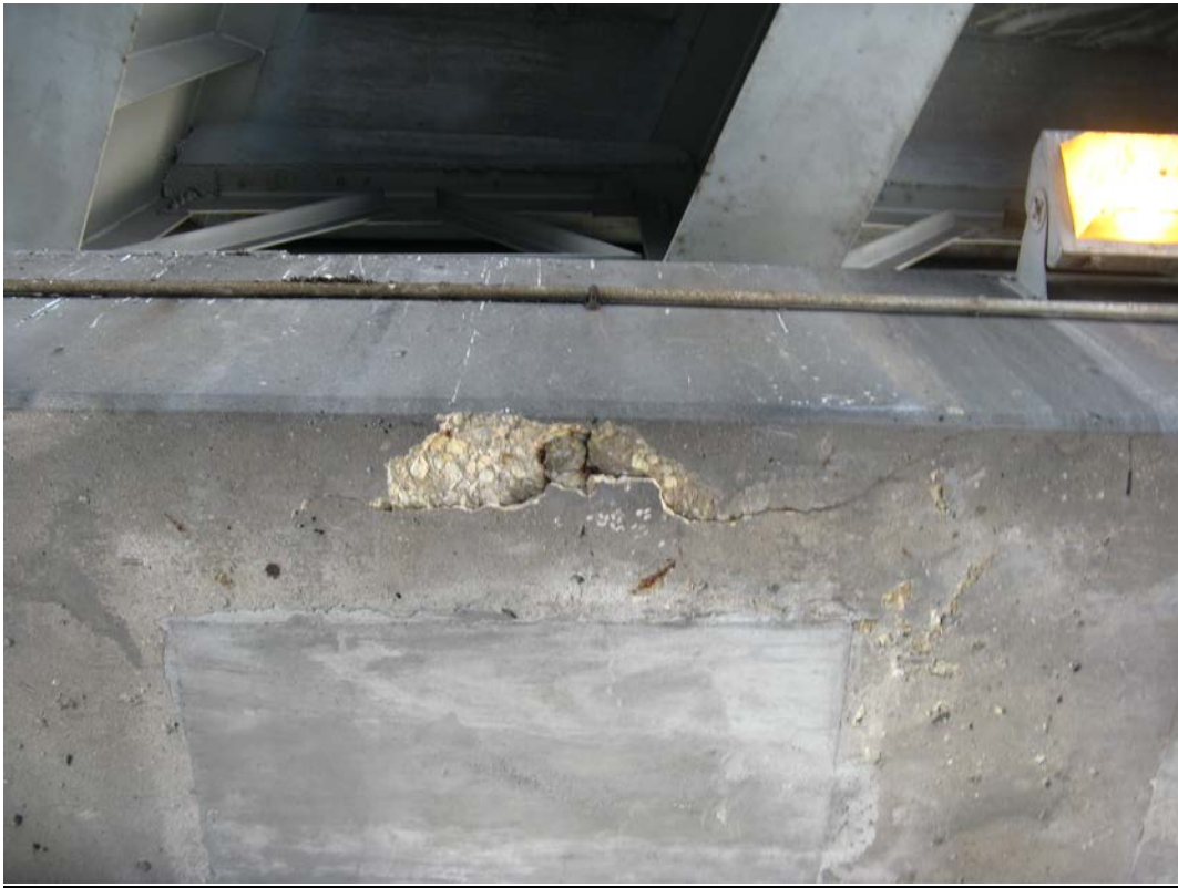
Photo 33 - East Pier, spall on underside of cap in between columns 3-4 from north, looking up and east
