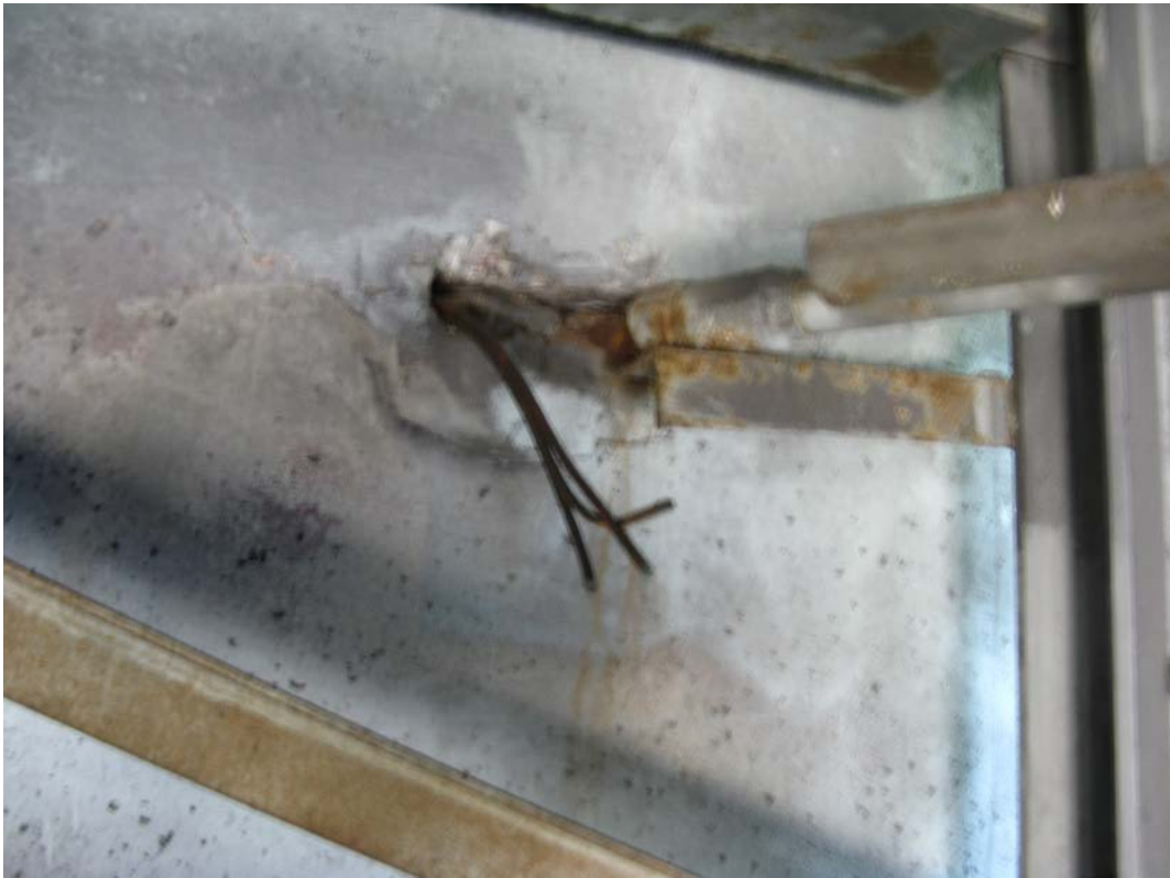
Photo 25 - Broken conduit at West Abutment backwall in bay 1 from north, looking west
