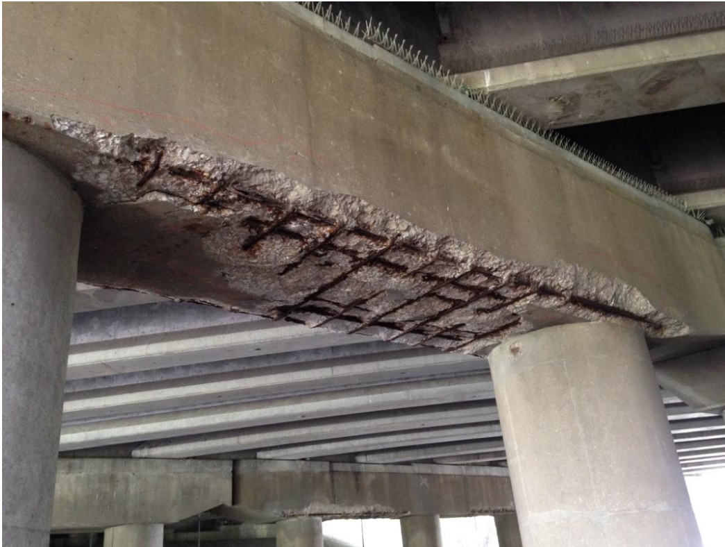
Photo 19: Pier 2, underside of pier cap between columns 10 & 11 showing spalling with exposed and corroded reinforcement.
