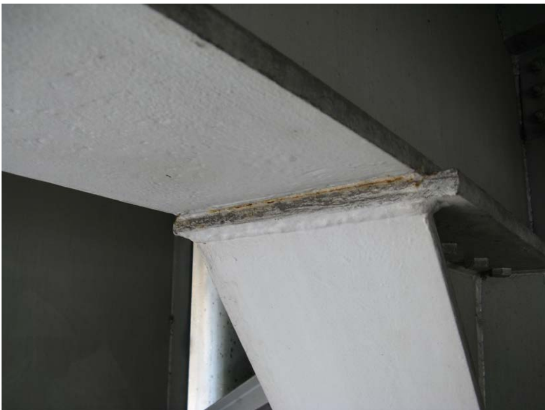
Photo 16 - Typical cracked weld between bottom flange of beam in east span and built up steel bolster, looking northeast (Beam 2 from north at East Abutment)
