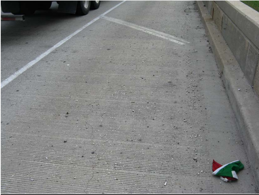
Photo 7 - Cracking in shoulder, Span 3, looking east
