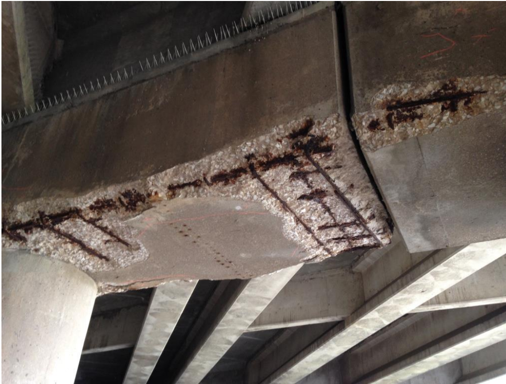
Photo 21: Pier 2, underside of pier cap between columns 3 & 4 showing spalling with exposed and corroded reinforcement on both sides of joint.
