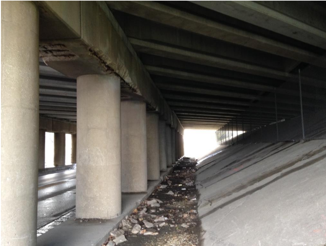
Photo 3: Span 1 overall looking south showing debris at base of east slopewall.
