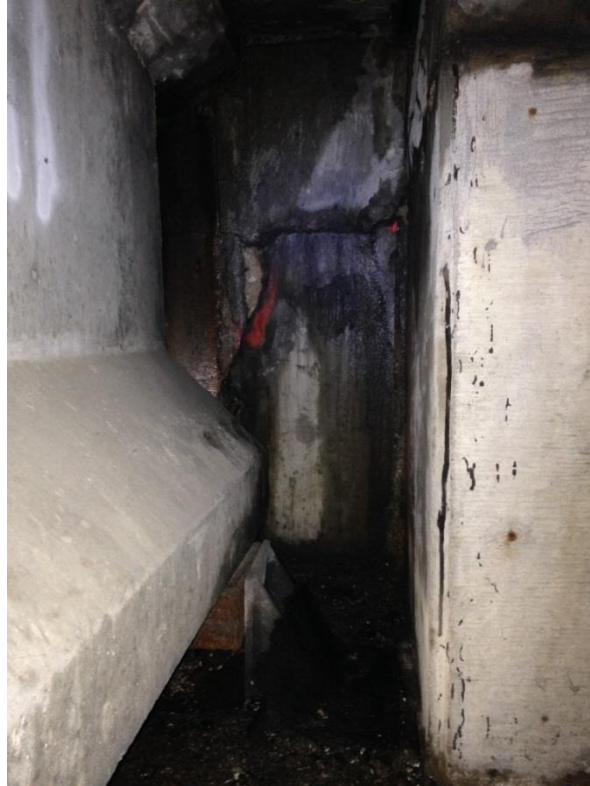
Photo 31: East abutment backwall at median joint showing water staining.
