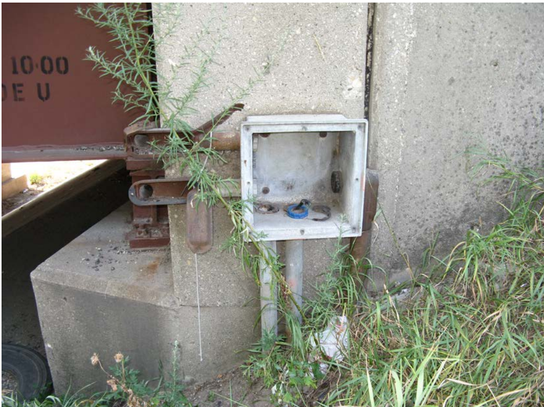
Photo 24 - Broken and open conduit on north end of West Abutment, looking south
