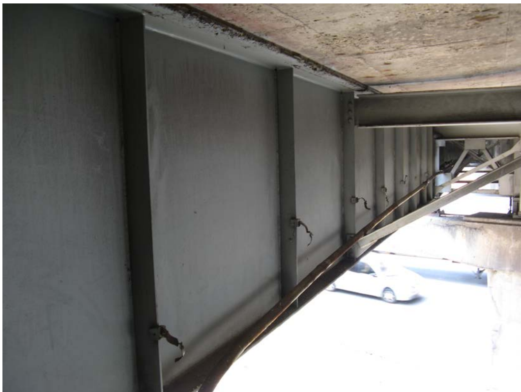
Photo 20 - Broken conduit from brackets along south fascia beam in Span 1, looking southwest
