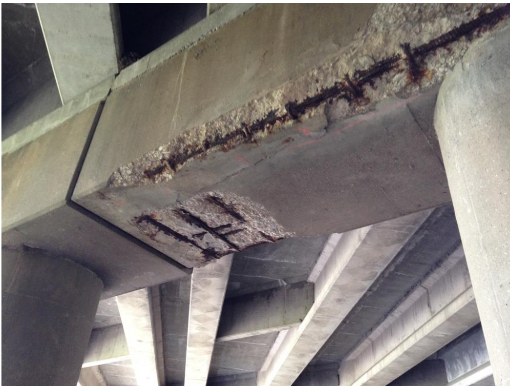
Photo 24: Pier 1, underside of pier cap between columns 3 & 4 showing spalling with exposed reinforcement on underside and bottom west corner of pier cap.
