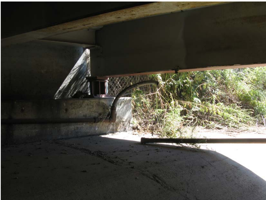
Photo 20 - Broken conduit on south side of Span 3, looking south
