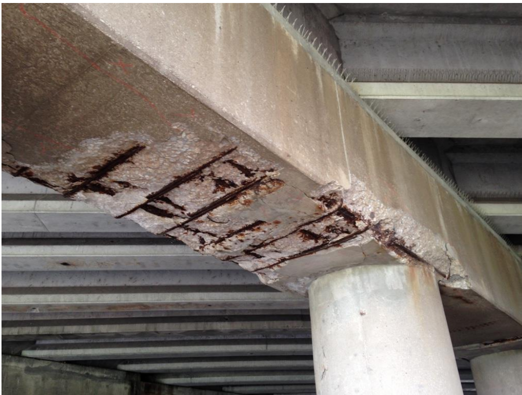
Photo 18; Pier 2, underside of pier cap between girders 12 & 13 showing spalling with exposed and corroded reinforcement.
