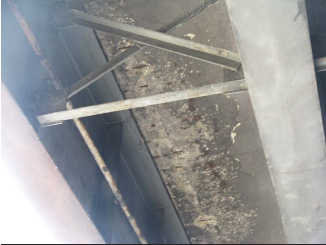
Photo 1 - Spalling in bay 9, Span 2 , east end, looking west
