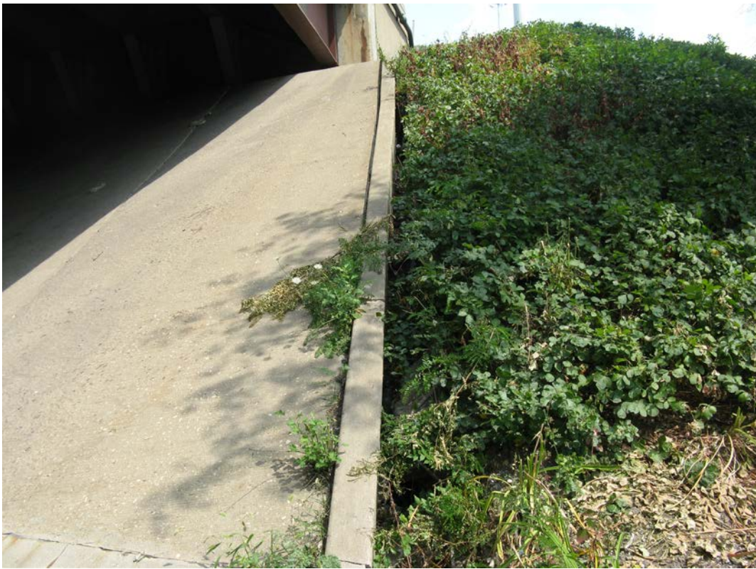
Photo 32 - Undermining of east sloped wall at south end, looking east
