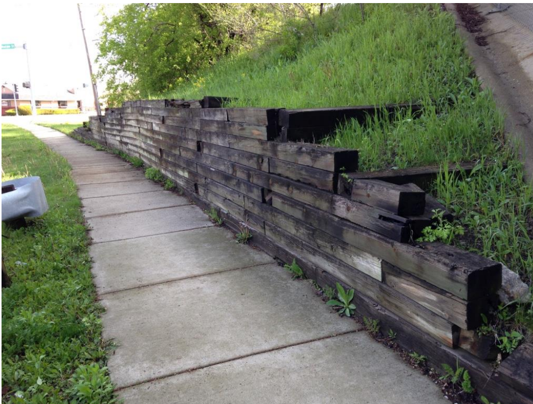
Photo 46: Timber tie-back retaining wall on the north east corner of the bridge starting at the base of the slope wall.
