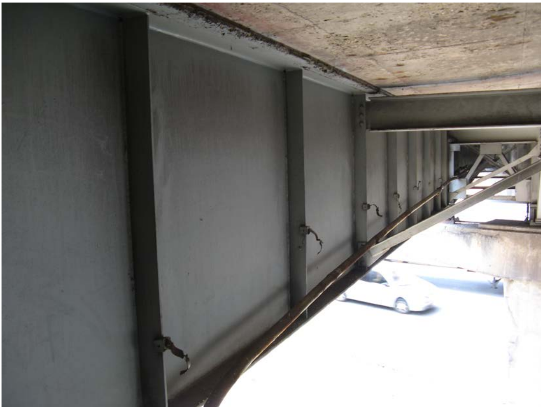
Photo 20 - Broken conduit from brackets along south fascia beam in Span 1, looking southwest
