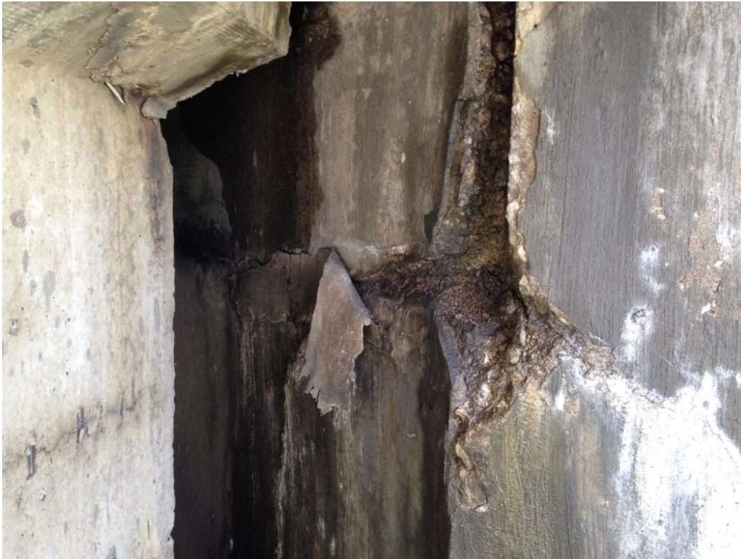
Photo 27: East abutment back wall south of girder 22 showing spall with loose crack seal and efflorescence.
