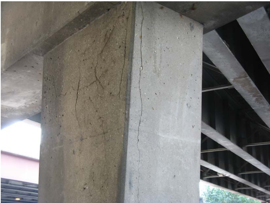
Photo 34 – East Pier, delam on northeast corner, looking southwest
