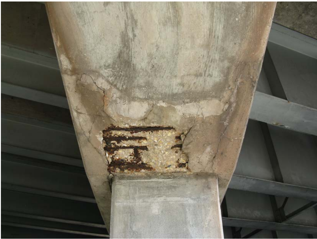
Photo 30 - Spall on underside of West Pier cap, south end, looking north
