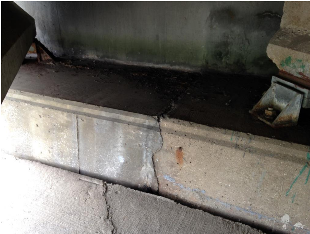
Photo 34: West abutment between girders 22 & 21 showing start of addition to abutment for widening.
