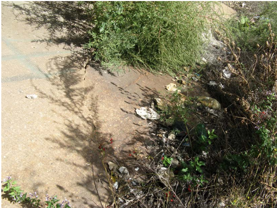
Photo 26 - Cracked west slopewall at southeast corner, looking east
