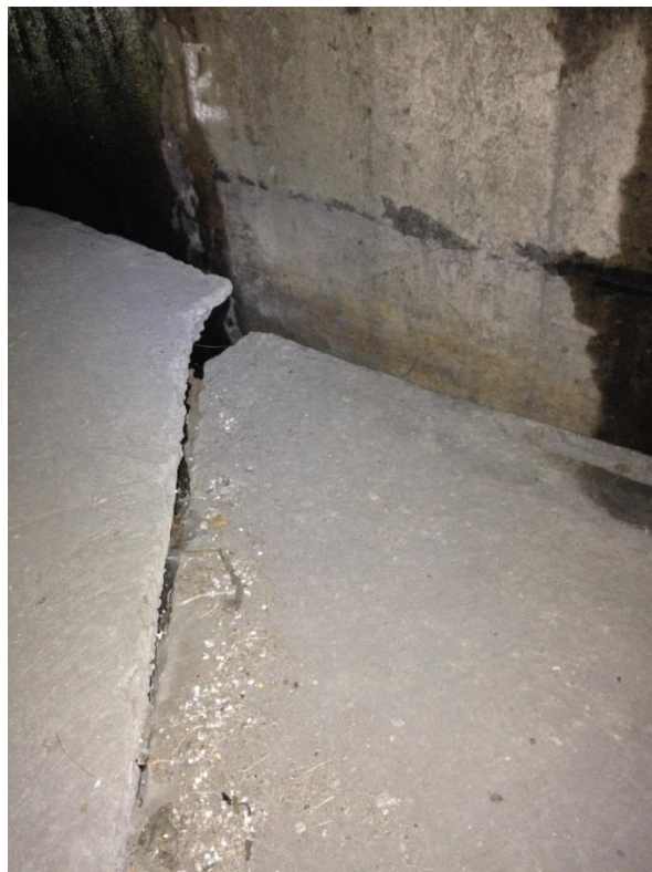
Photo 38: West abutment between girders 8 & 9 showing slope wall faulting with an offset of approximately 4 inches.
