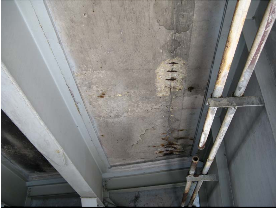
Photo 1 - Spalls on underside of deck in Span 3 between Beams 9-10 from north, east end, looking east
