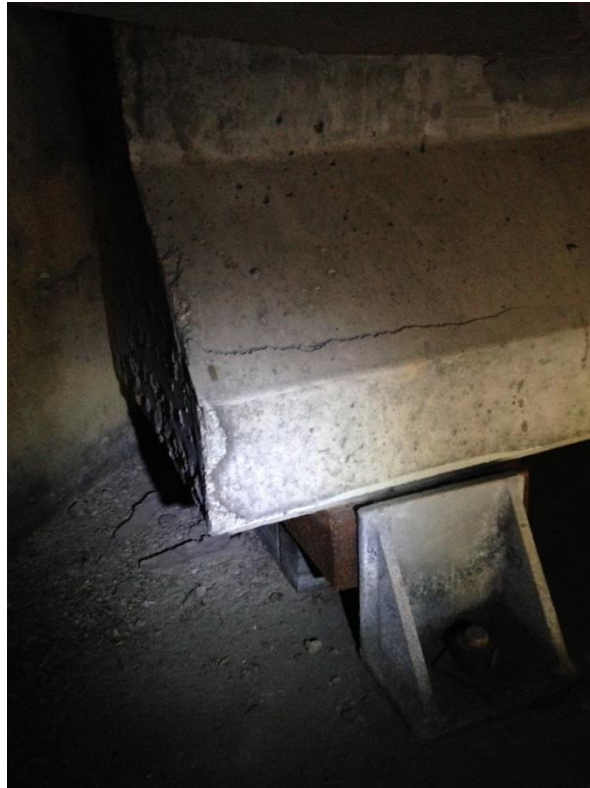
Photo 11: North face of girder 13 over east abutment showing area of delamination above bearing.
