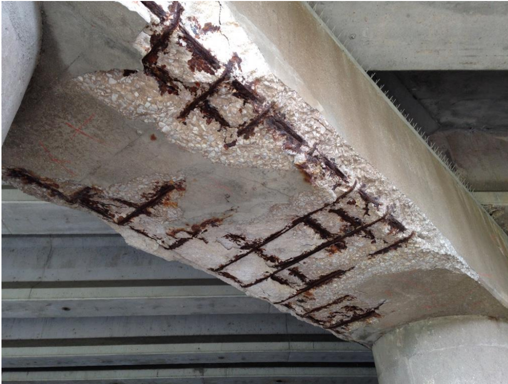
Photo 17: Pier 2, underside of pier cap between columns 13 & 14 showing spalling with exposed and corroded reinforcement.
