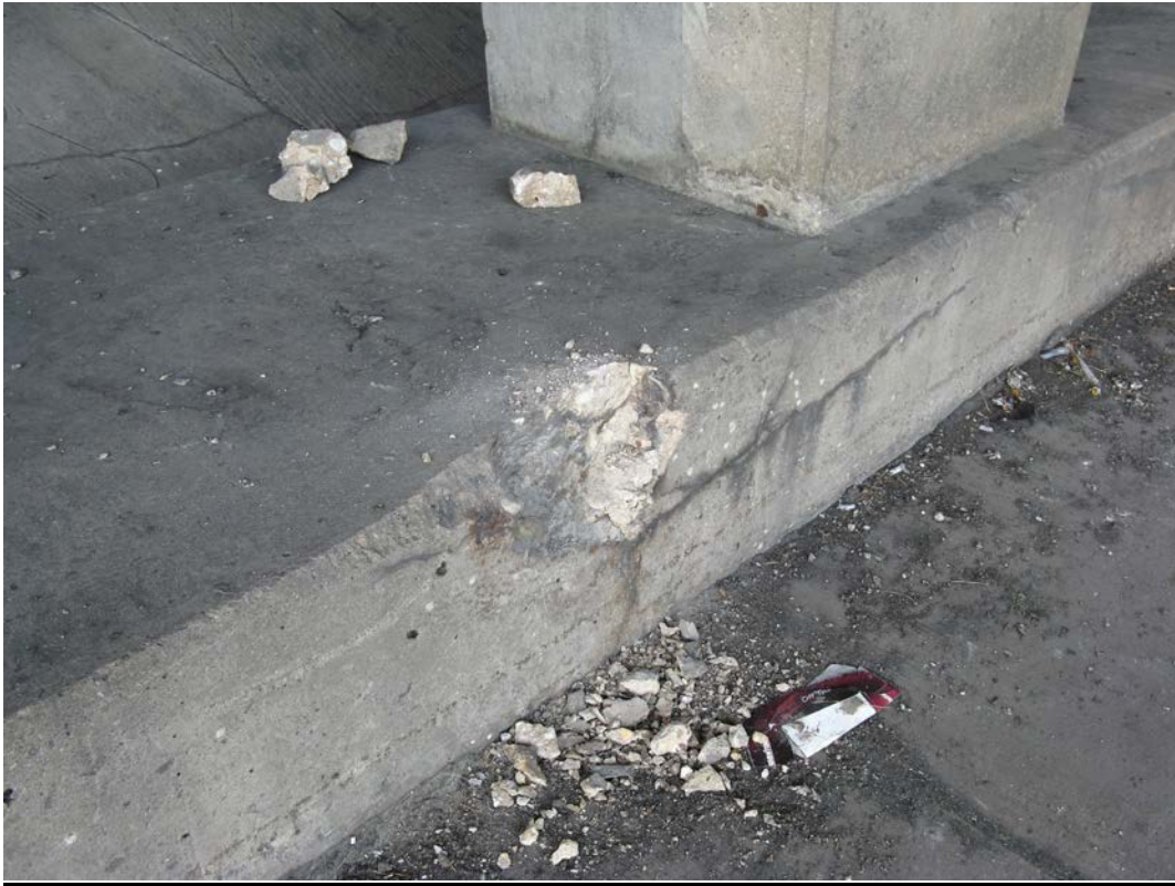
Photo 35 - Spall in East Pier crashwall, north of second column from north, west face, looking southeast
