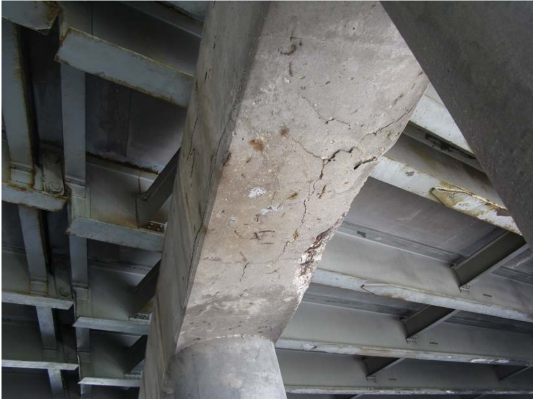
Photo 23 - Delaminated and spalled underside of Pier 1, looking northeast
