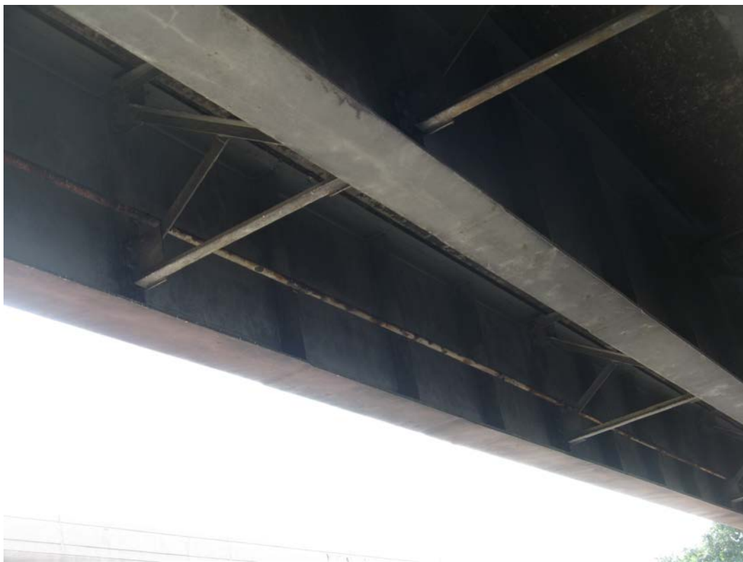
Photo 19 - Failed conduit connections, looking southwest
