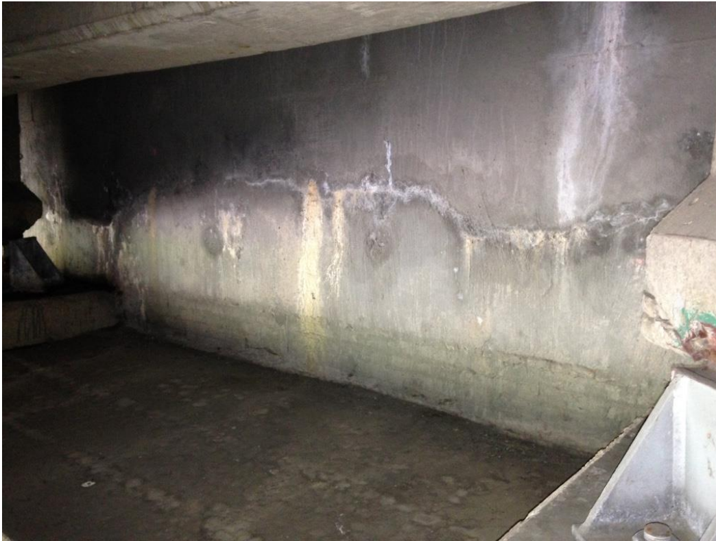
Photo 37: West abutment between girders 14 & 15 showing cold joint with efflorescence on backwall.
