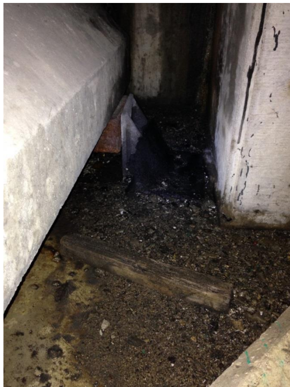
Photo 32: East abutment seat at median joint showing sediment build-up.
