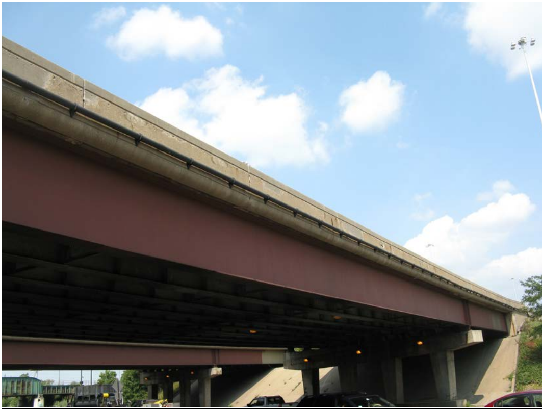
Photo 9 - Outside of South Parapet with minor rust stains, cracking, and minor spalling, looking northeast
