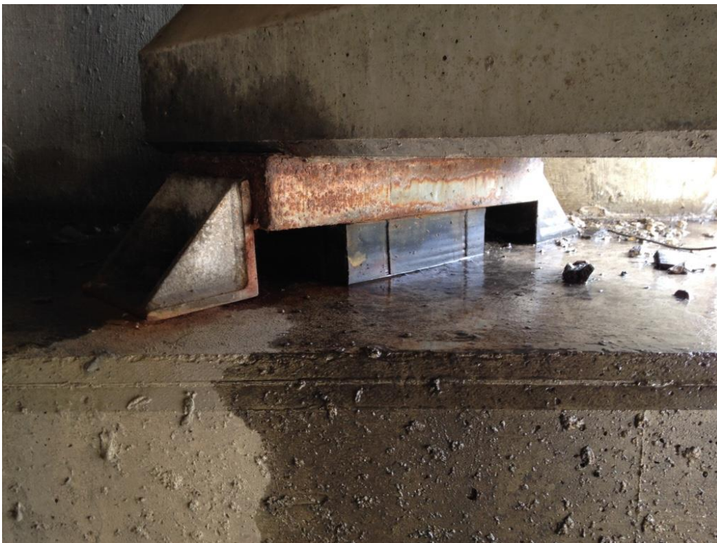
Photo 28: East bearing under girder 22 (typ.) showing standing water near backwall and corrosion of bearing top plate.
