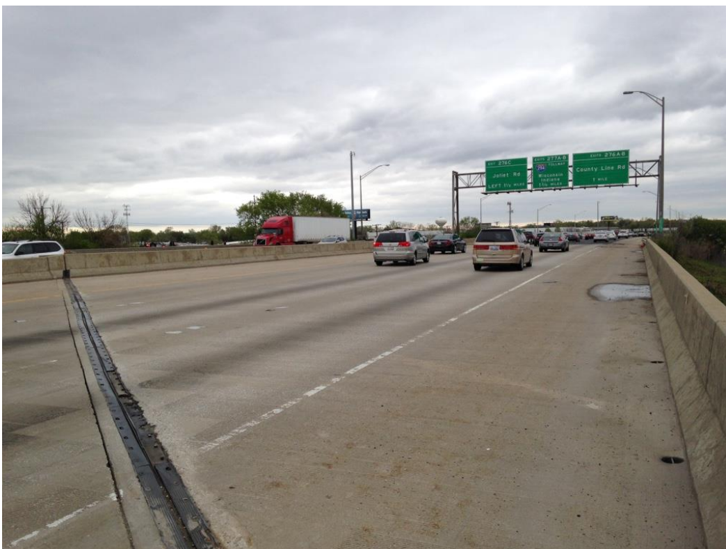
Photo 2: Top of deck looking east from southwest corner, ponding near midspan of south parapet.
