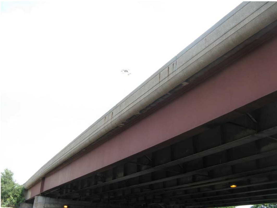
Photo 10 - Outside of North Parapet with minor rust stains and cracking, looking southeast
