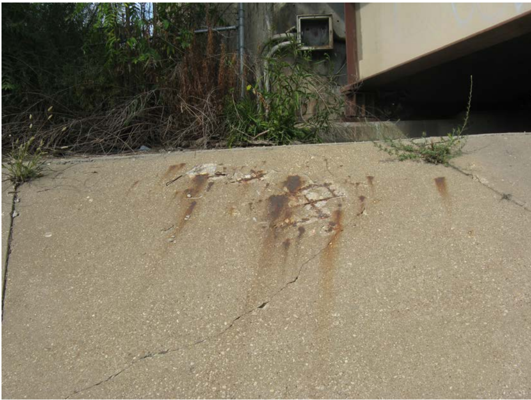
Photo 40 - Spall in west sloped wall, looking west
