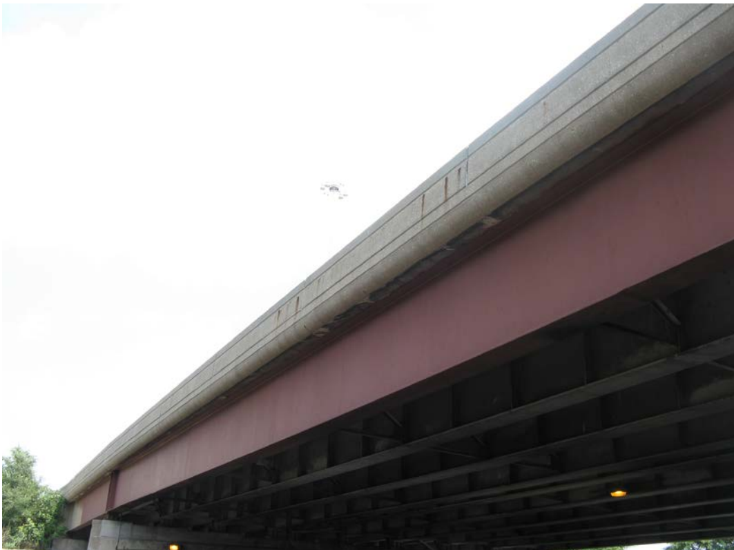
Photo 10 - Outside of North Parapet with minor rust stains and cracking, looking southeast
