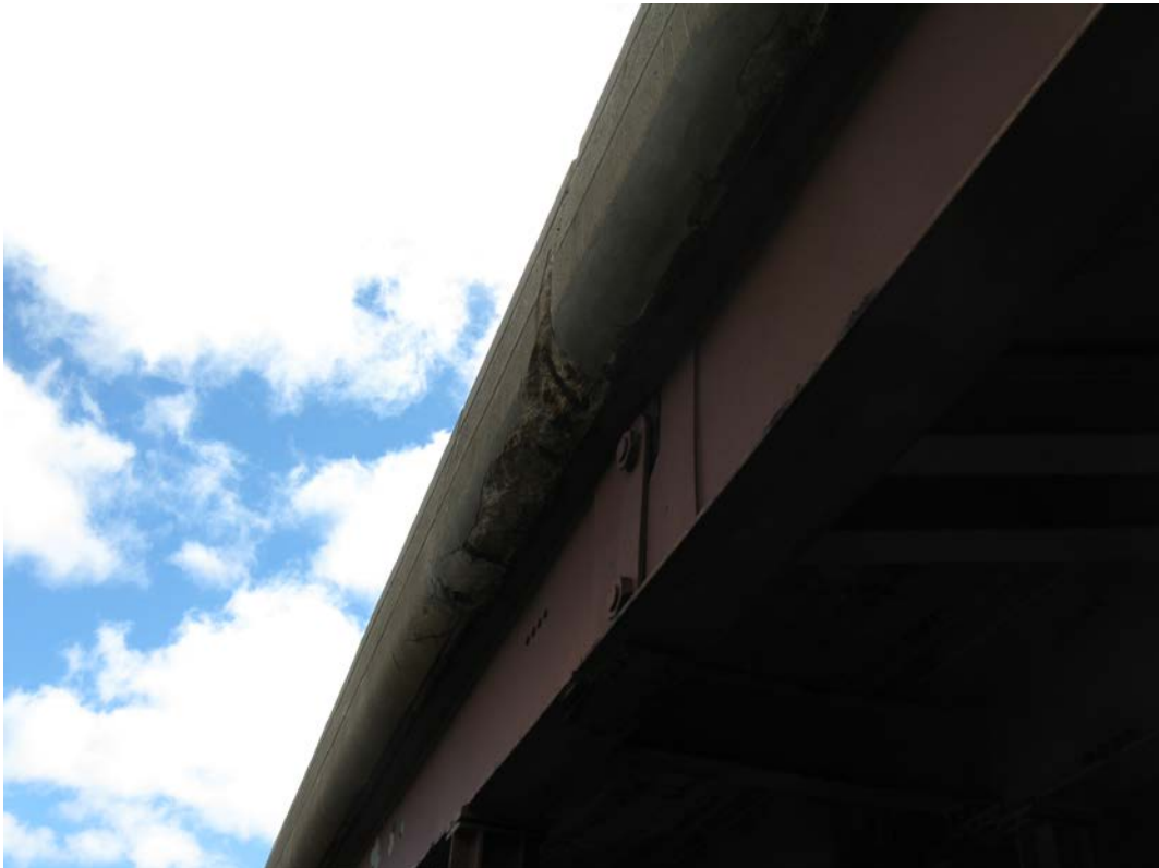
Photo 8 - Spalled parapet at north side at Span 1, looking southeast
