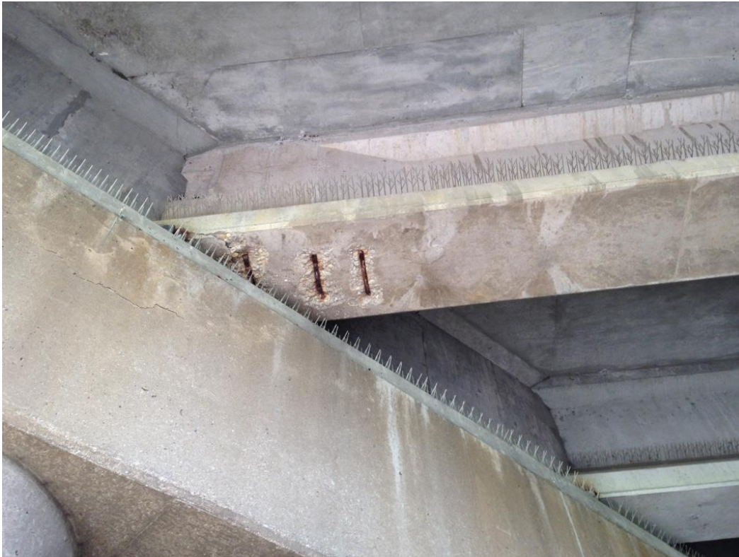
Photo 7: Span 3, underside of girder 19 at pier 2 showing spalling with exposed and corroded stirrups.
