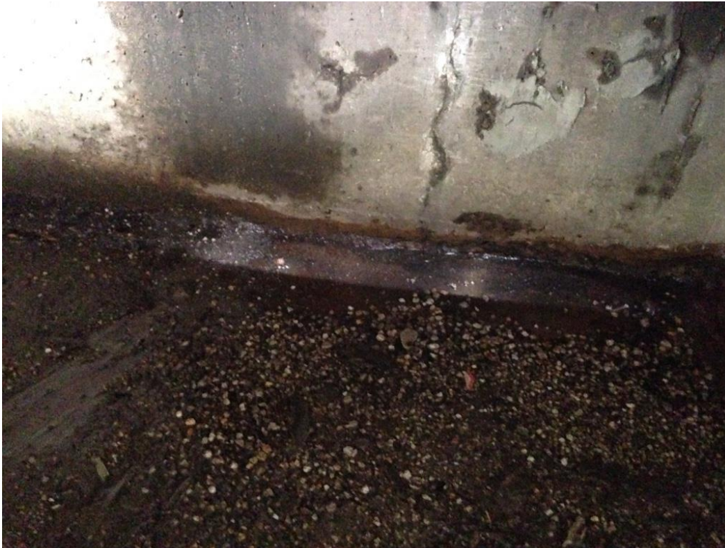
Photo 29: East abutment between girders 19 & 20 showing sediment deposit on abutment seat and light coming through from the top of deck due to missing joint section above.
