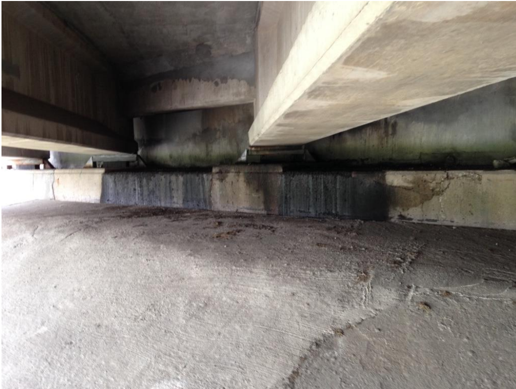
Photo 35: West abutment between girders 20 & 21 showing water staining on abutment seat.
