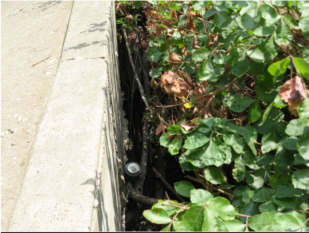
Photo 31 - Undermining of east slopewall at south end, looking east
