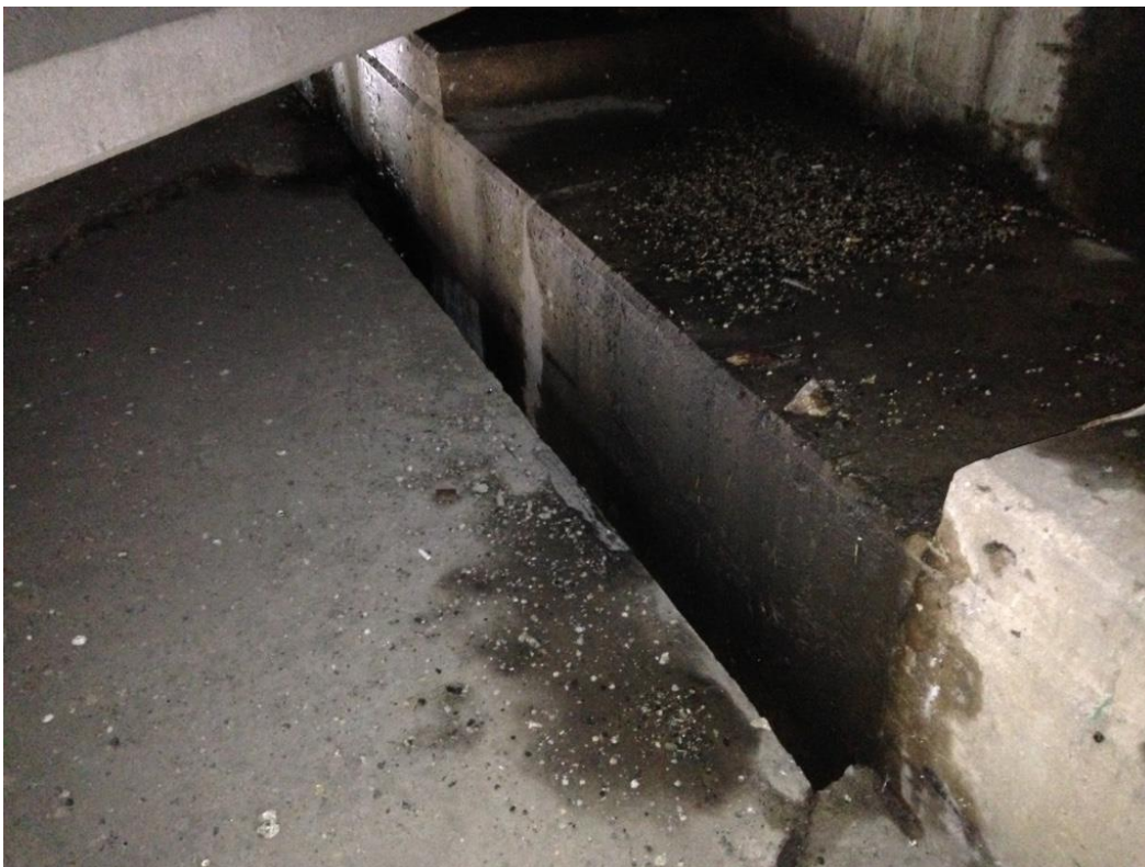
Photo 30: East abutment between girders 14 & 15 showing approximately 3.5 inch separation of slopewall from abutment seat.
