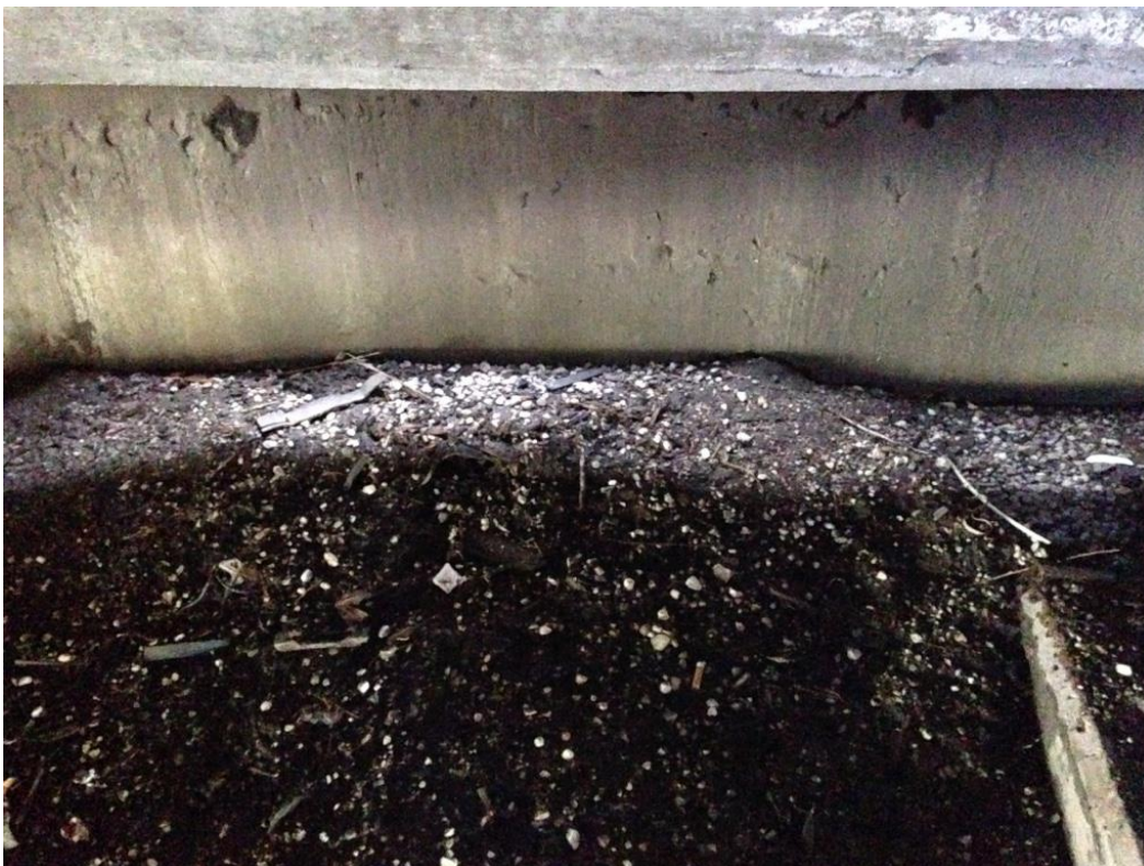
Photo 40: West abutment between girders 3 & 4 showing deposit of sediment and light coming through from top of deck due to missing joint section above.
