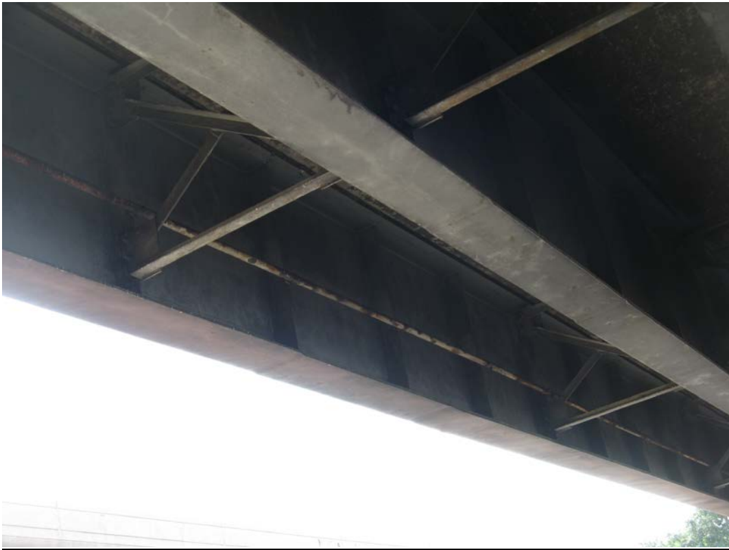
Photo 19 - Failed conduit connections, looking southwest
