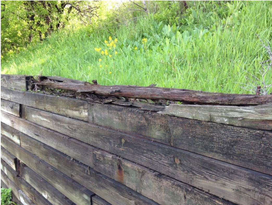
Photo 47: Splitting top members on retaining wall.
