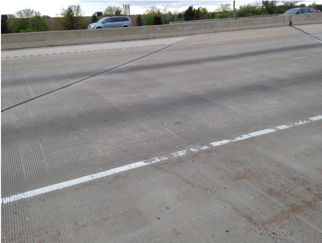
Photo 51: North west approach slab looking south showing hairline cracking.
