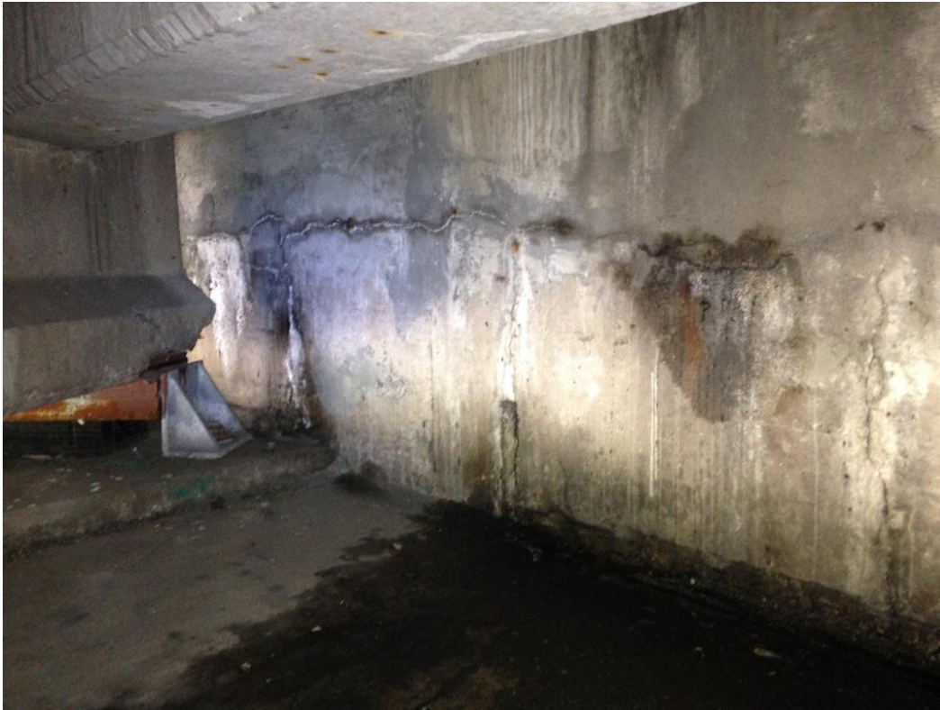
Photo 33: East abutment between girders 7 & 8 showing cold joint with efflorescence on backwall and water staining on abutment seat.
