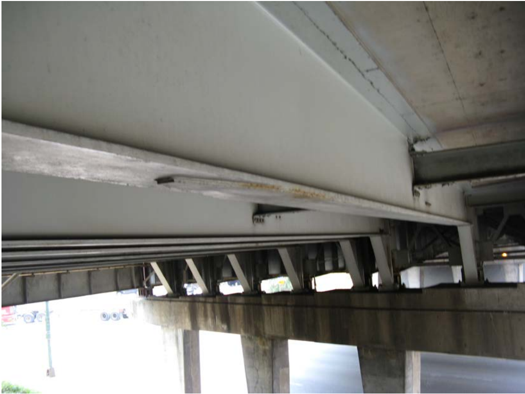
Photo 17 - Typical cover plates on bottom on beams in east span, looking southwest (Beam 3 from north, Span 3)
