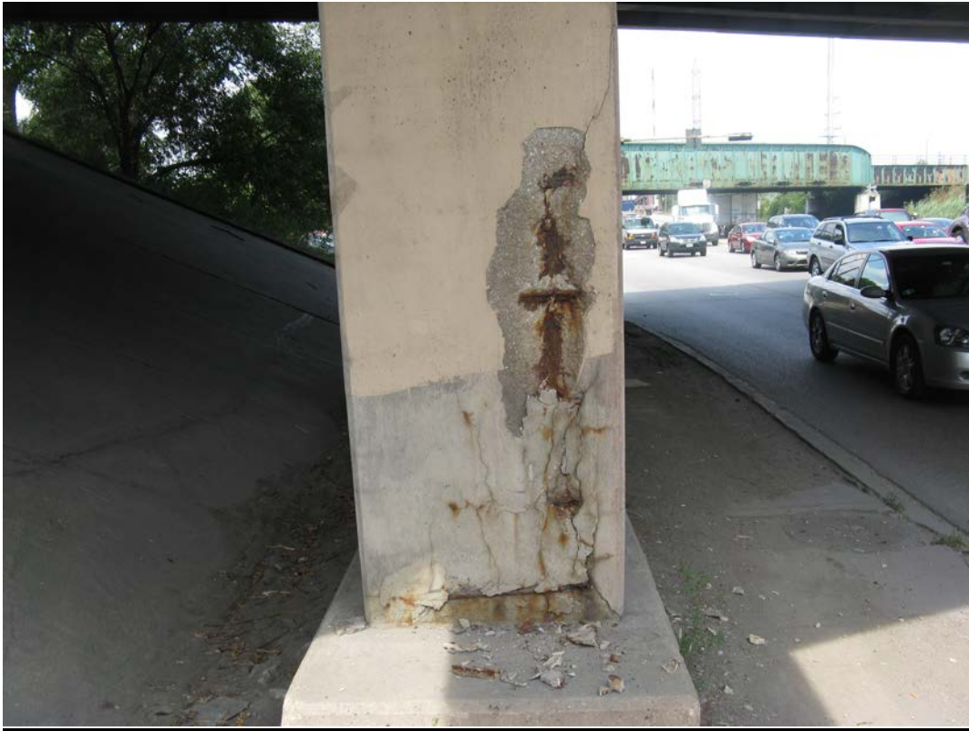
Photo 37 - Spall on West Pier, south face, bottom of fourth column from north, looking north
