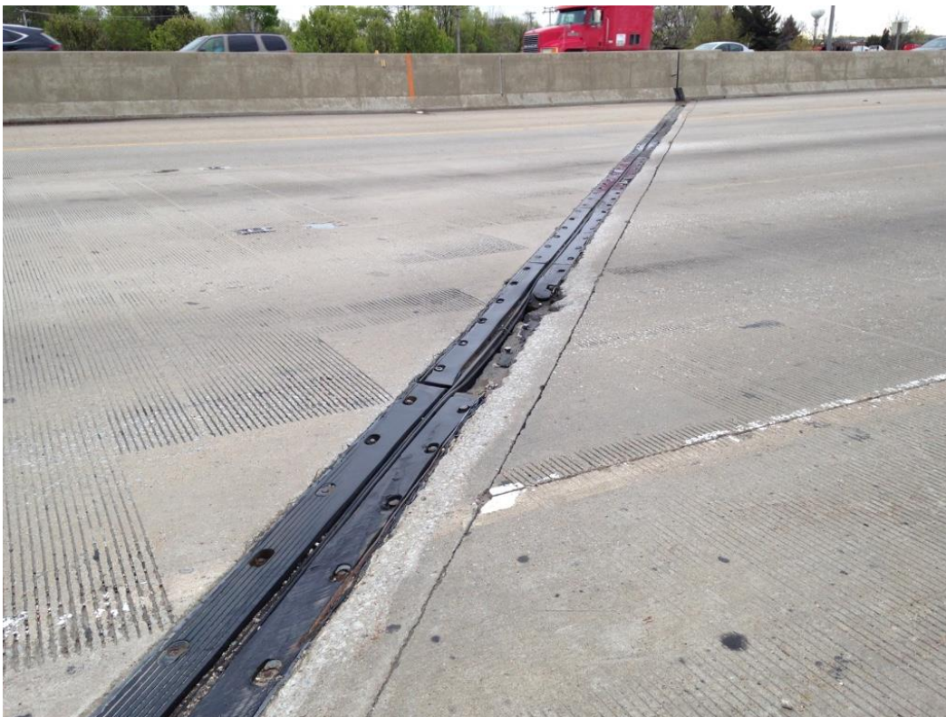
Photo 50: Transverse joint on north west end of bridge, looking south showing missing sections, exposed steel bolts, and abrasion damage to approach slab concrete.
