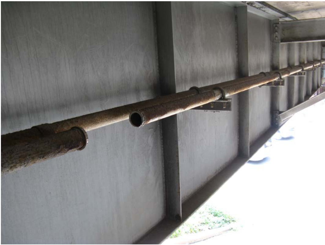
Photo 20 - Broken conduit along South Fascia Beam, Span 3, 8' from East Abutment, looking west
