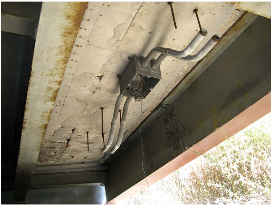
Photo 18 - Abandoned utility box in Span 3, southern most bay
