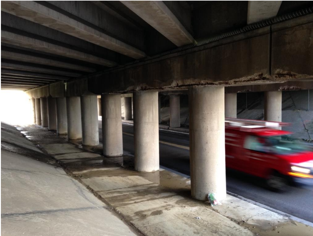
Photo 15: Pier 2 overall looking southwest showing build-up of mud on sidewalk.
