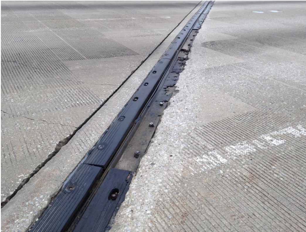
Photo 49: Transverse joint on the south west end of the bridge, looking north showing missing sections, exposed steel bolts, abrasion damage on bridge deck concrete and hairline cracking on approach slab.
