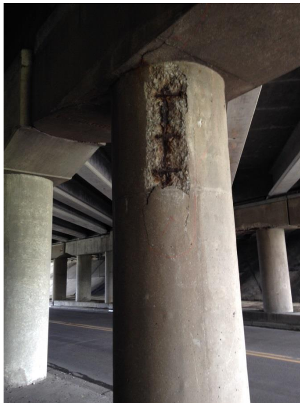
Photo 22: Pier 1, southwest face of column 10 showing spalling with exposed and corroded reinforcement near the pier cap.
