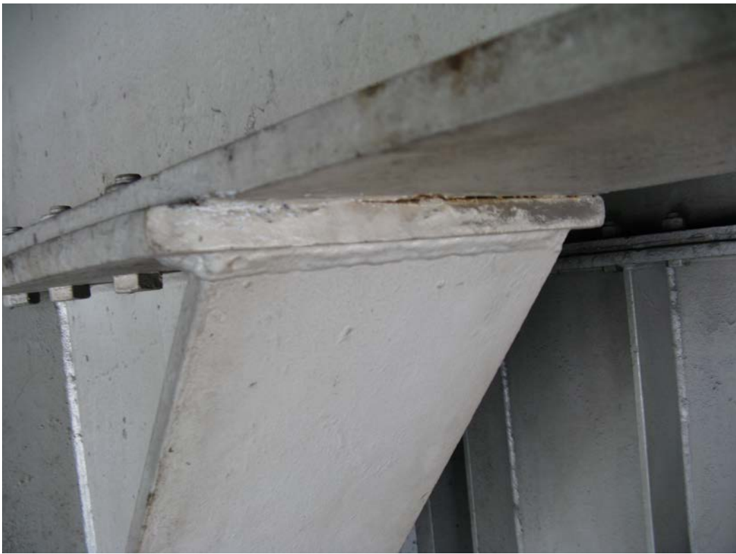
Photo 14 - Typical cracked weld between bottom flange of beam and built up steel pedestal, Beam 6 at East Abutment, looking southeast
