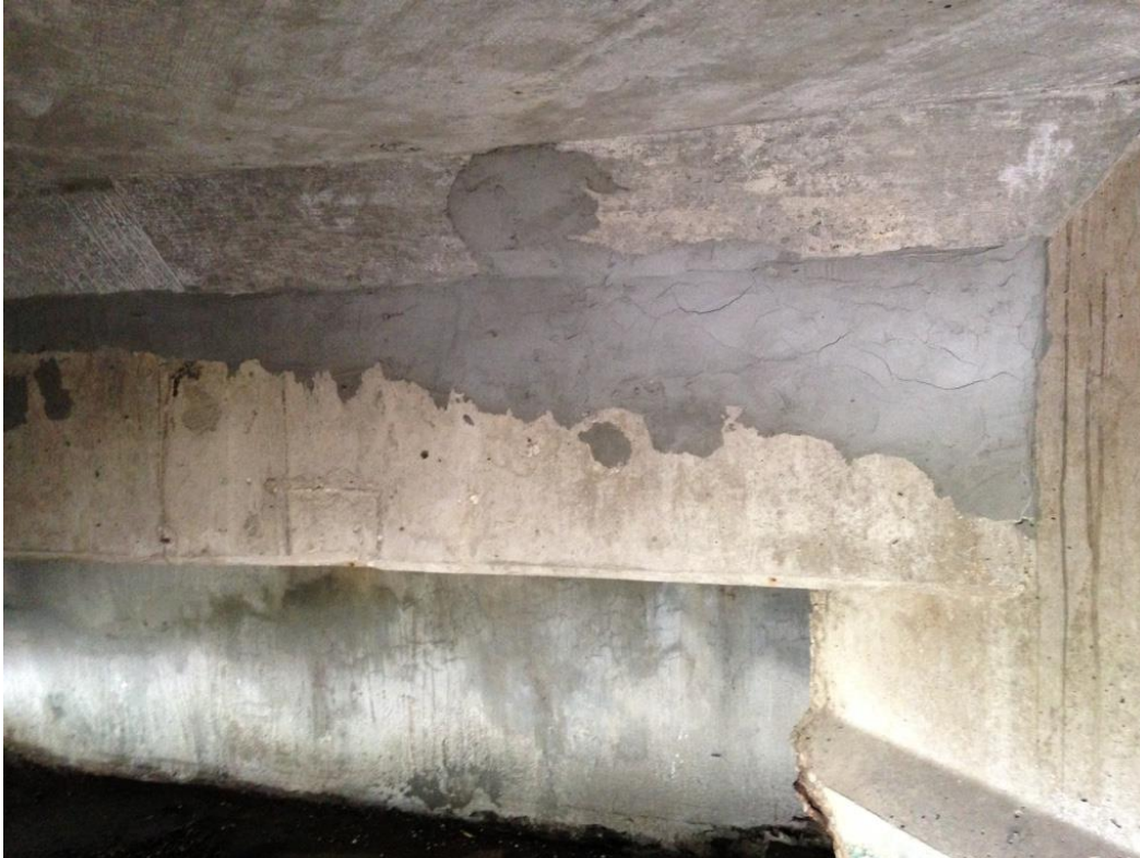
Photo 9: Diaphragm between girders 21 and 20 at west abutment showing previously patched area intact.
