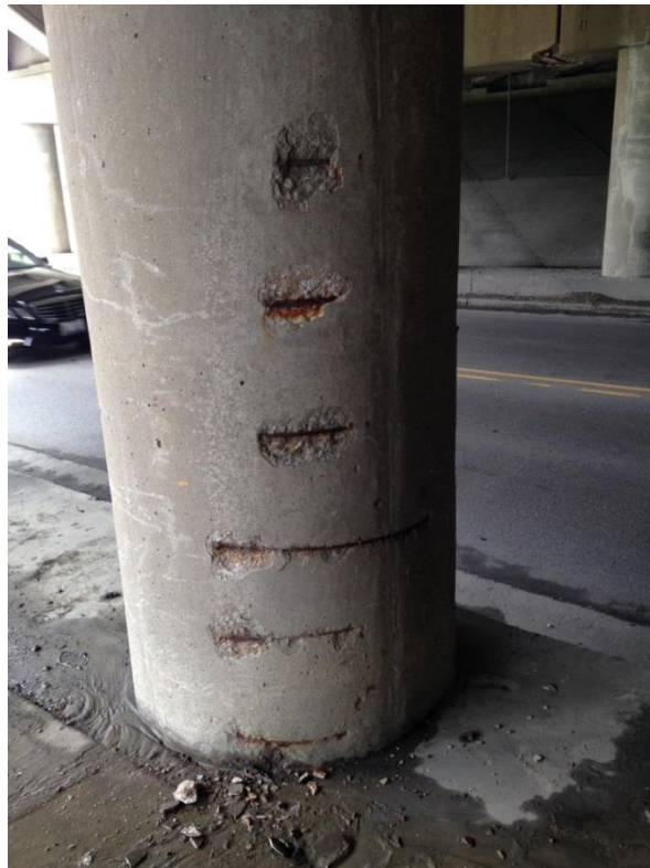
Photo 20: Pier 2, north east face of column 14 showing exposed and corroded spiral reinforcement.
