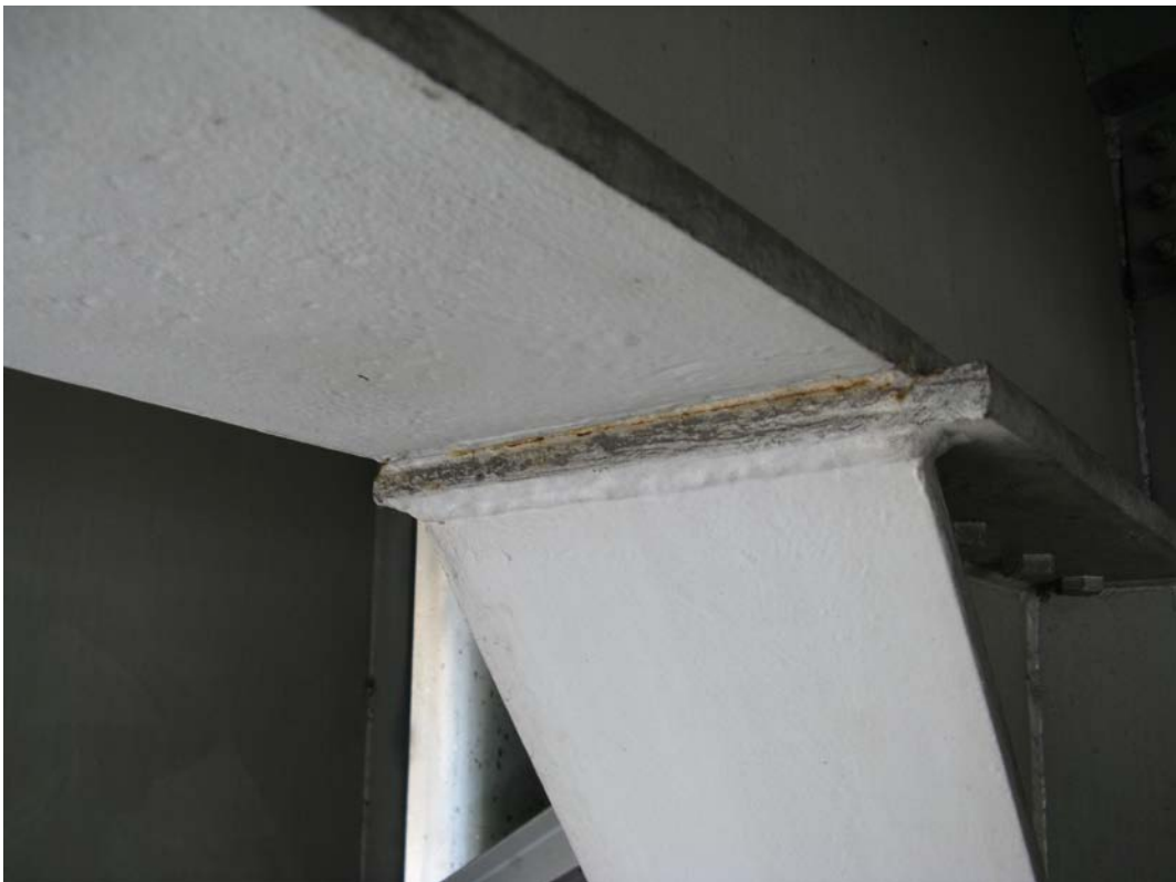
Photo 16 - Typical cracked weld between bottom flange of beam in east span and built up steel bolster, looking northeast (Beam 2 from north at East Abutment)
