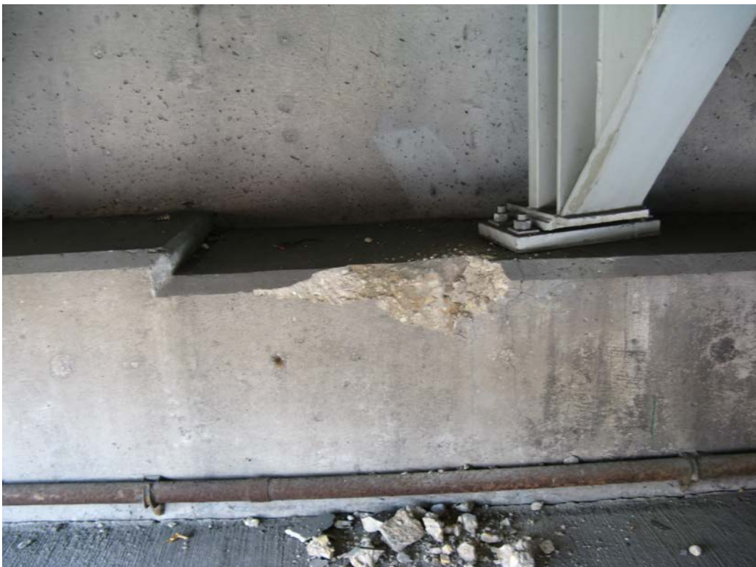
Photo 22 - Spall on East Abutment seat between beams 2-3, looking east
