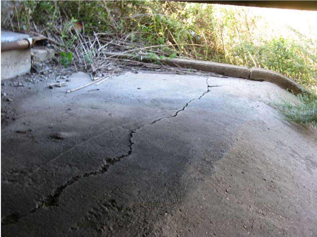
Photo 27 - Crack at Span 1 sloped wall, looking northwest
