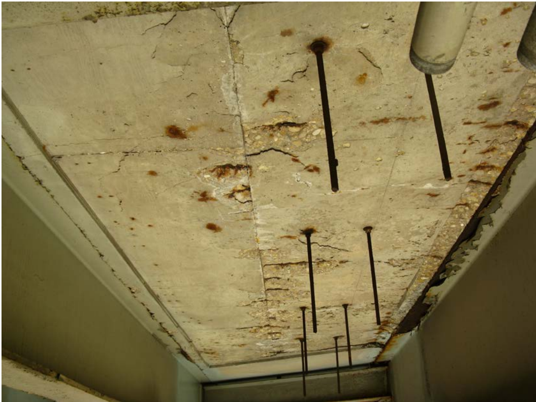
Photo 1 - Delaminated underside of deck at south side of Span 1
