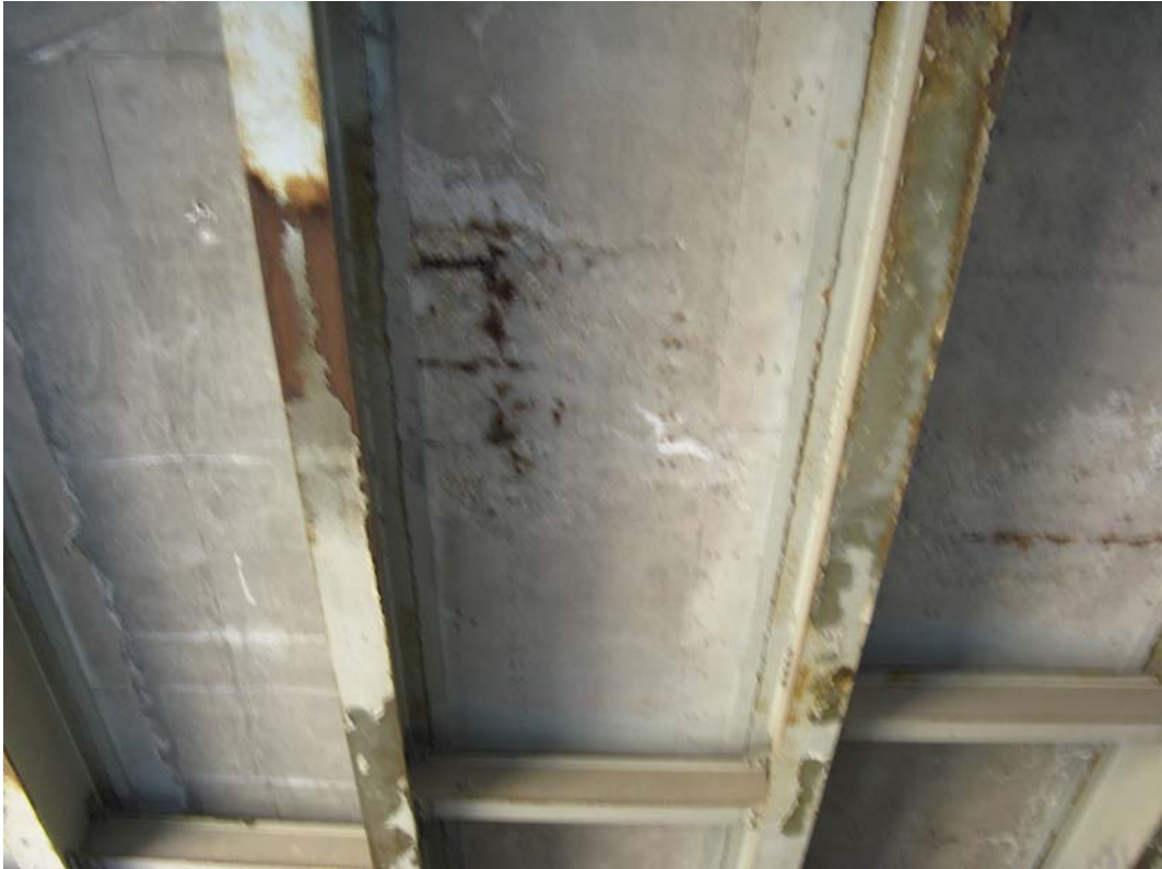
Photo 3 - Deteriorated concrete in Span 1, looking west
