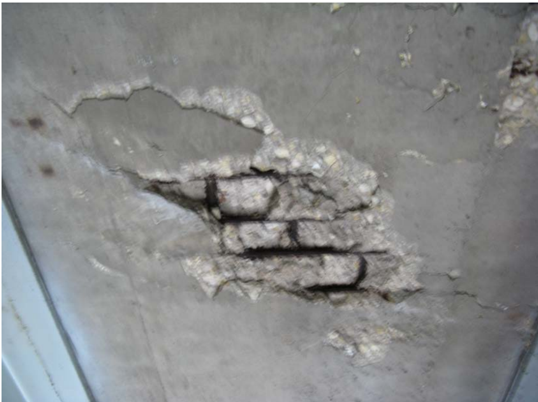
Photo 2 - Spall underside of deck in Span 3, east end, between beams 1-2 from north, looking west
