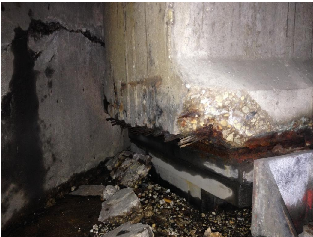
Photo 10: East end of girder 19 showing spalled bottom cover with exposed and corroded bottom row of prestressing strands.
