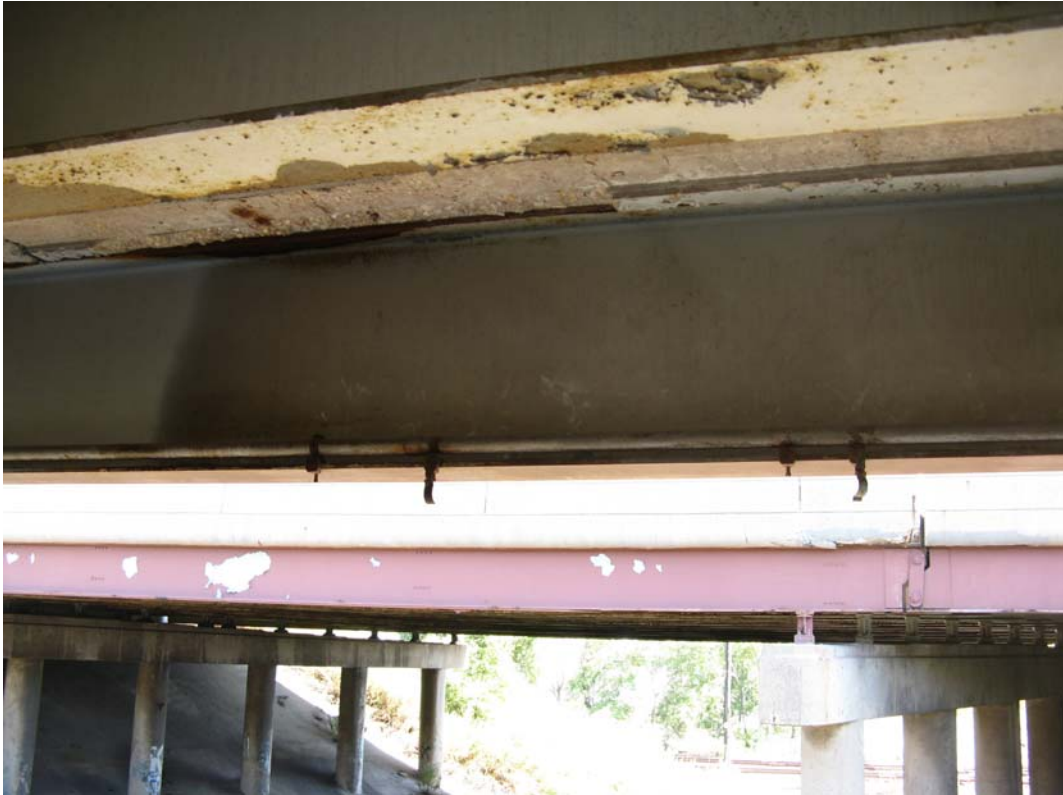
Photo 21 - Broken brackets on conduit, looking south
