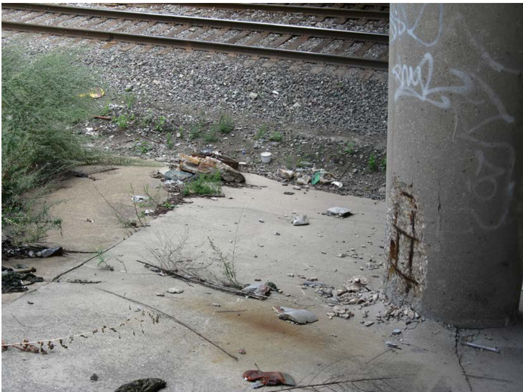
Photo 24 - Spalled column at Pier 1
