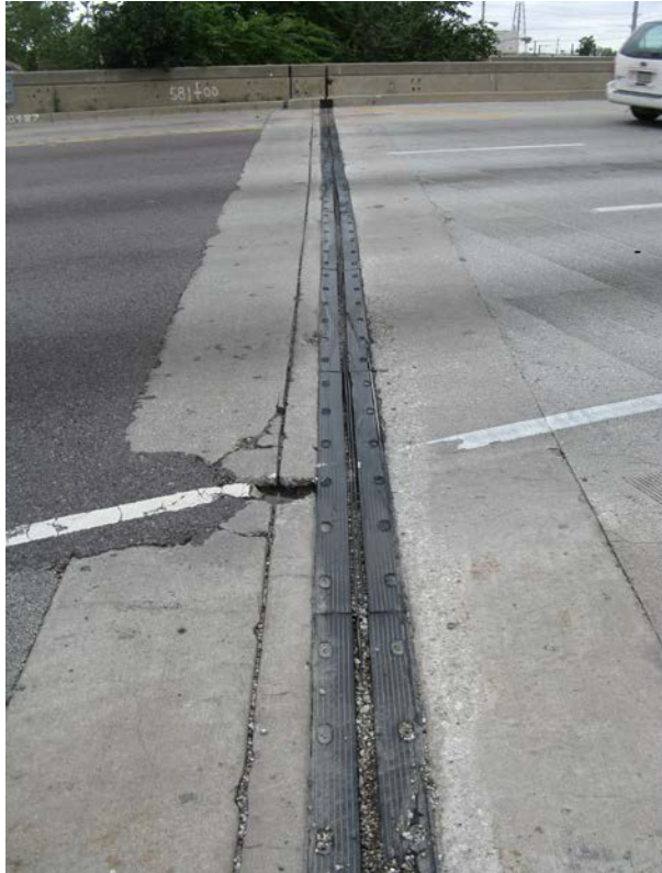
Photo 11 - West Abutment joint, looking north
