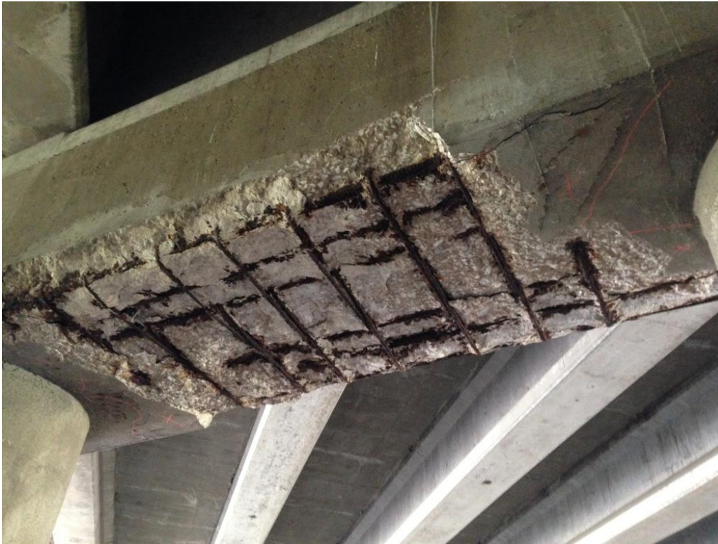
Photo 23: Pier 1, underside of pier cap between columns 5 & 6 showing spalling with exposed and corroded reinforcement.
