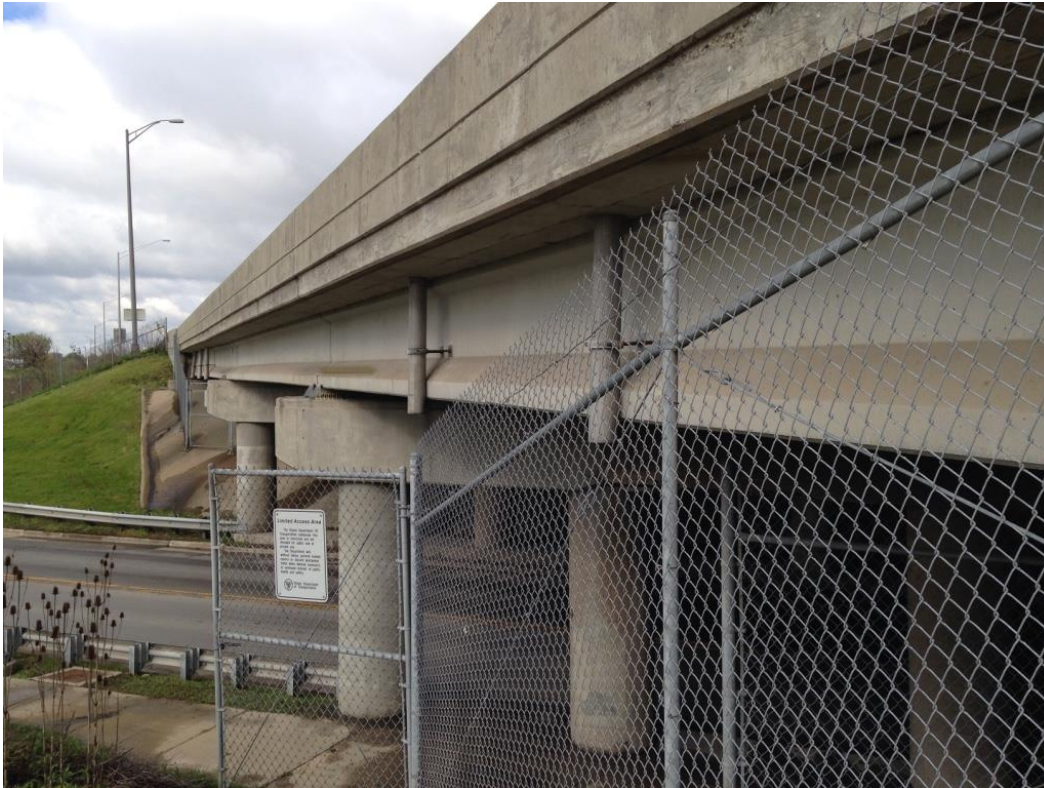
Photo13: South side of structure looking southwest along fascia showing deck drain down spouts.
