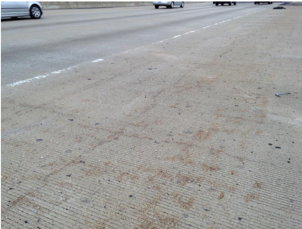
Photo 52: Top of deck on north end of bridge, looking west showing hairline longitudinal and transverse cracks on shoulder.
