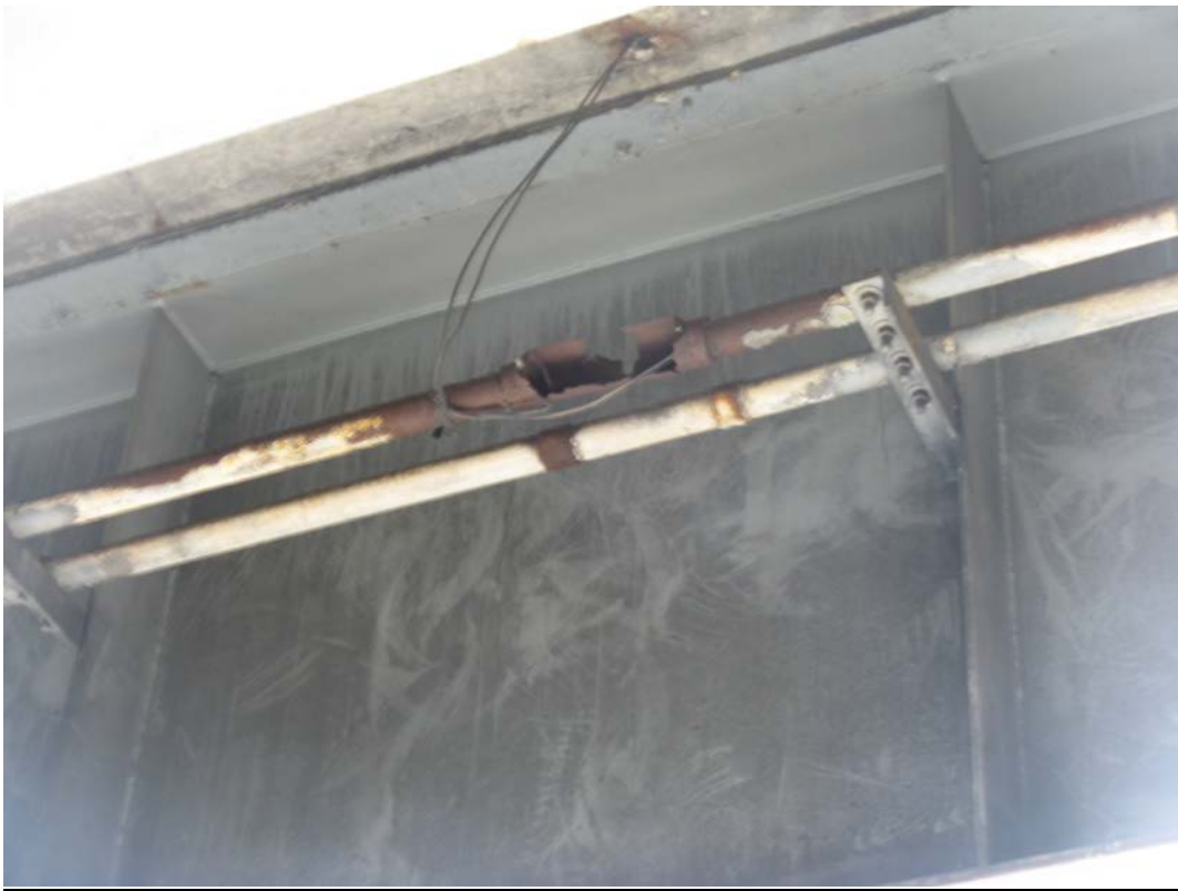
Photo 21 - Broken conduit in Span 2 along south fascia beam, 6' from West Pier, looking southeast
