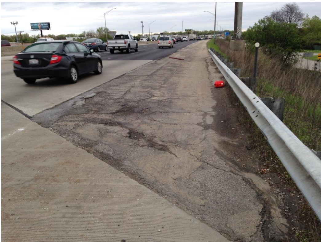
Photo 48: Top of deck looking east showing shoulder just beyond east approach slab showing significant cracking and potholes.
