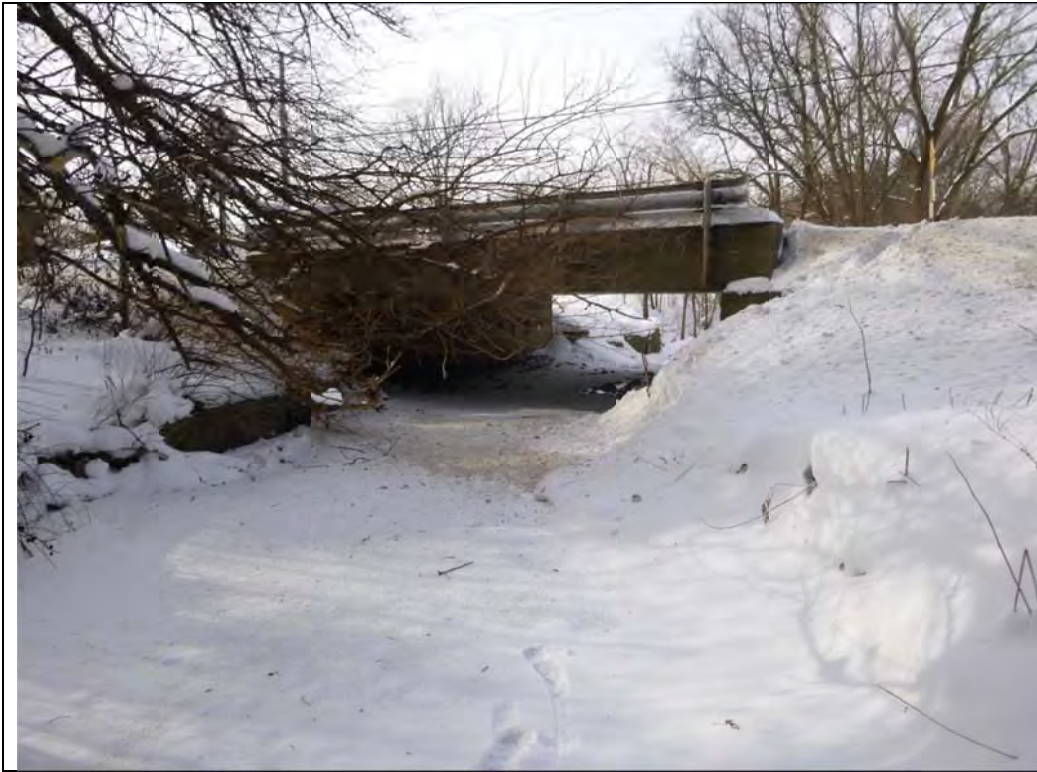
Photo #8 – Structure Upstream of Project: Clarendon Hills Road Bridge - Upstream Face (Looking West)
