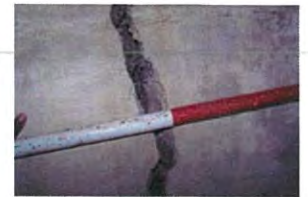
Culvert-Full Depth Crack at S
