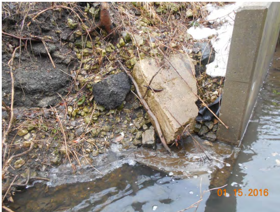
Photo 6: Northeast wingwall with footing exposed due to scour.
