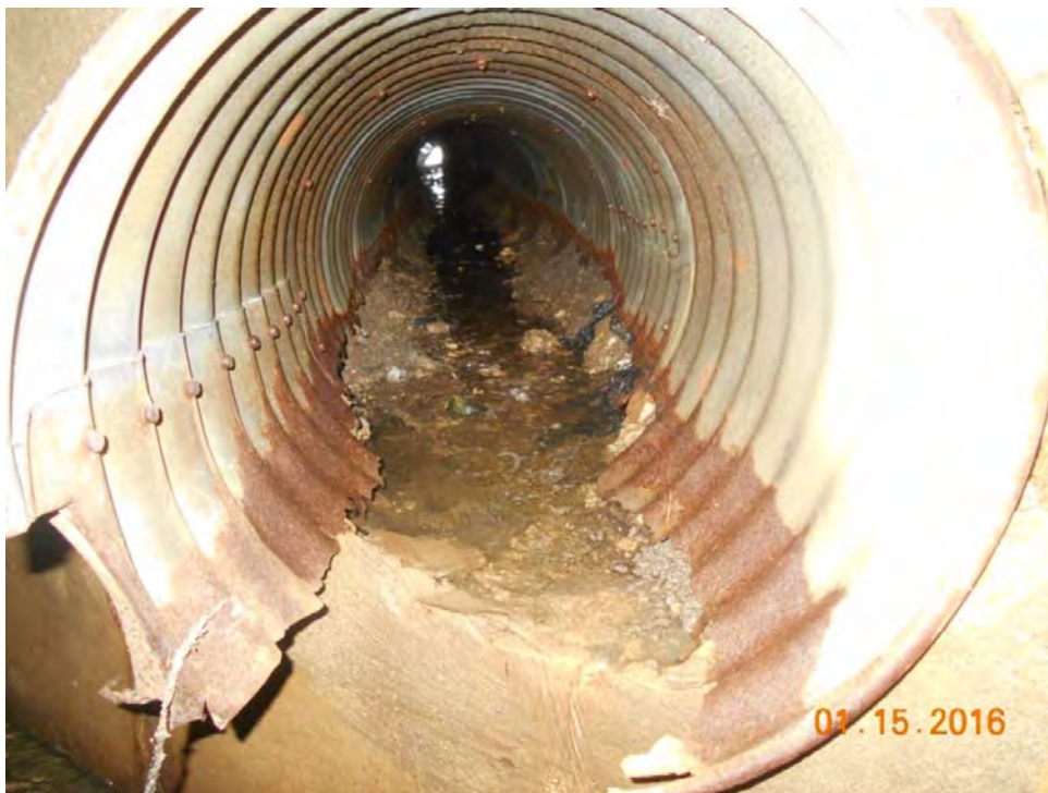
Photo 4: Severely corroded CMP in west wall near the south end of culvert. Typical at other CMP locations.
