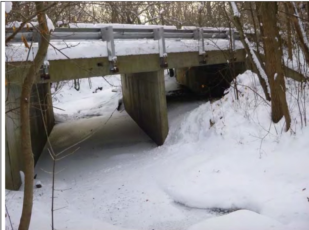
Photo #11 – Structure Downstream of Project: Western Avenue Culvert - Downstream Face (Looking East)
