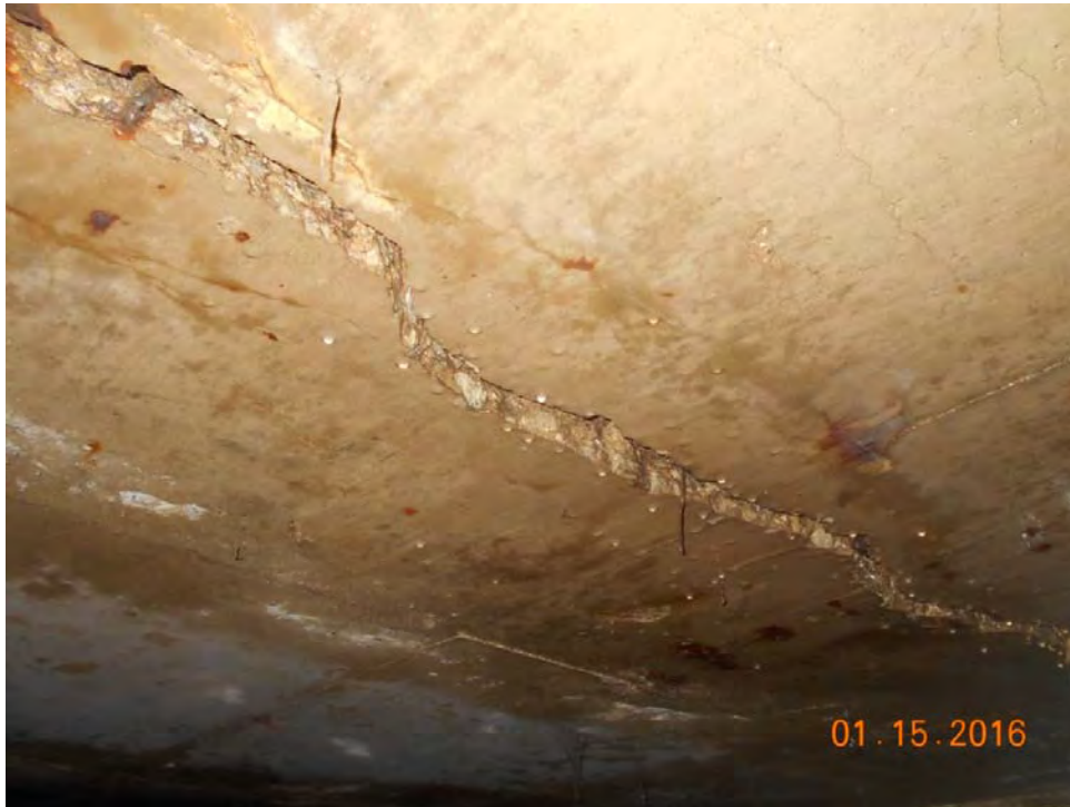
Photo 1: Underside of top slab showing large crack through top slab at south end.
