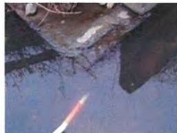
18 - Scour issue undermining NE WW.jpg
