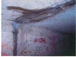
06 - Longit crack w water seeping and rust.jpg
