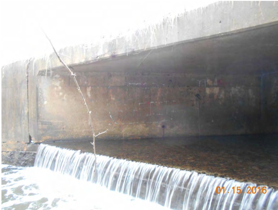
Photo 7: South end of culvert showing scour.
