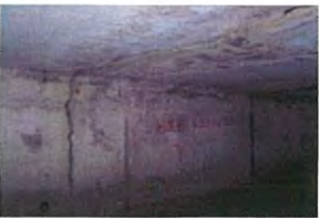
Culvert-Full Depth Crack at S Enc
