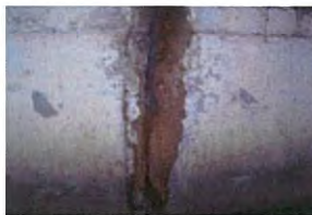
0017_Culvert-Longit crack with
