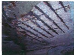
12 - Central section major spall w primary reinf expos...
