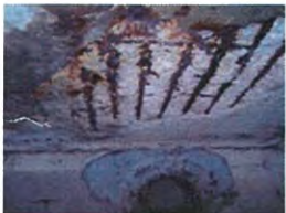
11 - Central section major spall w primary reinf expos...
