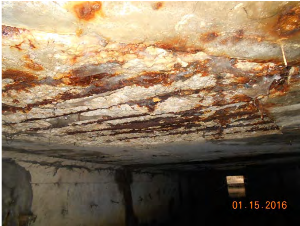
Photo 5: Underside of the top slab with large spall, center of culvert.
