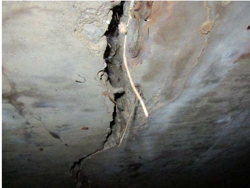
Figure 3. Large cracks in top slab and walls. Similar cracks observed approximately 50 ft. from each end.
