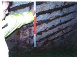
13 - Central section major spall w primary reinf expos...
