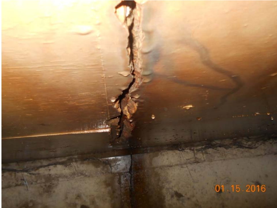
Photo 3: Underside of top slab showing large crack at north end.
