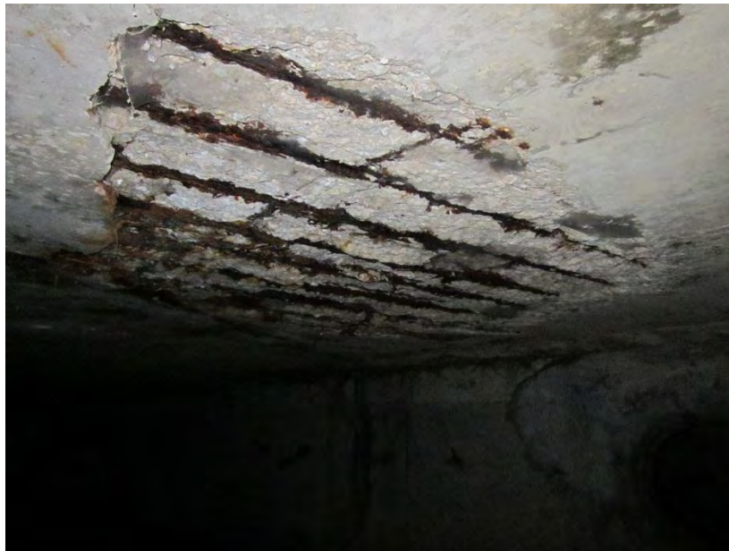
Figure 2. Large spall with exposed, corroding reinforcing bar near the median of I-55.
