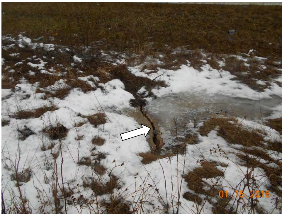
Photo 2: Large crack in top slab of culvert at south end visible in ditch of I-55.
