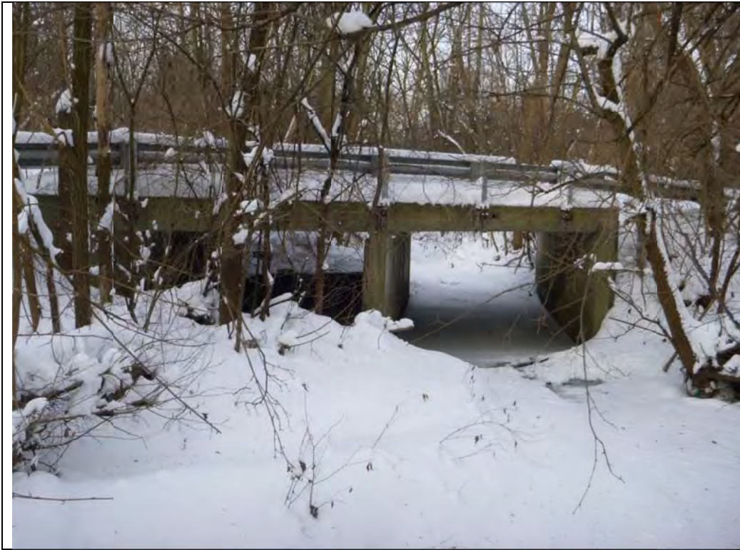
Photo #10 – Structure Downstream of Project: Western Avenue Culvert - Upstream Face (Looking West)
