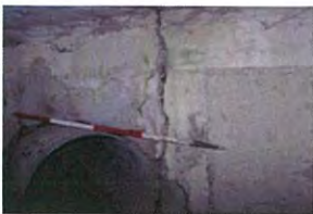
Culvert-Full Depth Crack at S En
