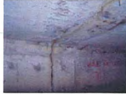
08 - Full depth crack at S end total separation.jpg
