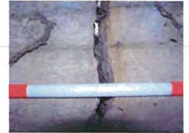
10 - Full depth crack at S end total separation.jpg.jpg
