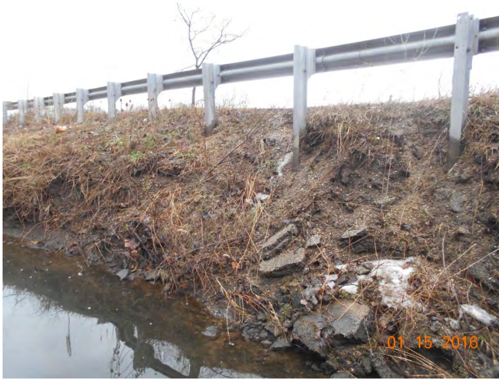
Photo 9: Slope failure at northeast wingwall.
