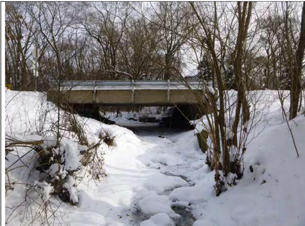
Photo #9 – Structure Upstream of Project: Clarendon Hills Road Bridge - Downstream Face (Looking East)
