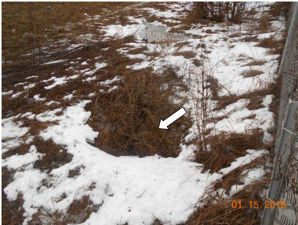
Photo 8: South I-55 ditch showing erosion. Top and side of culvert is visible under grass.
