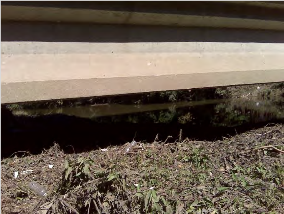
17. Debris pileup under 70 th Place Bridge, looking South downstream
