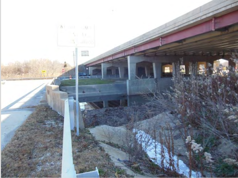
22. Paved ditch outlet to Flag Creek along South side of 70 th Place looking east.
