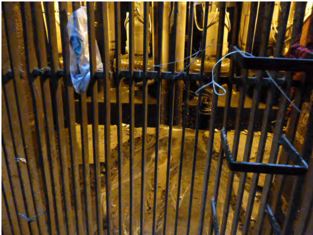
11. PS 30, trash rack and pumps in wet well
