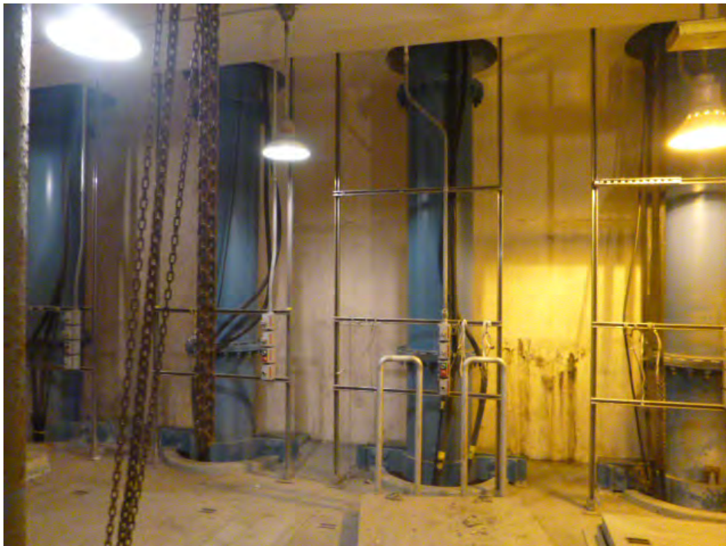
7. PS 30, pump room, intermediate floor, looking east
