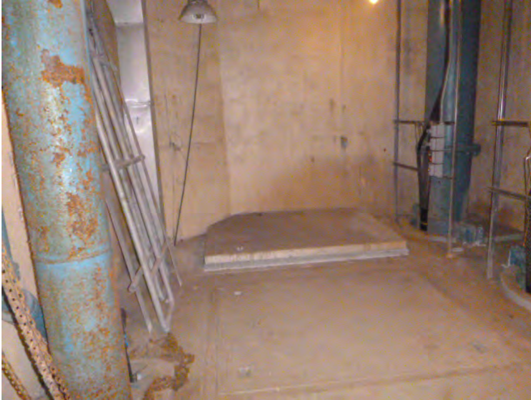
6. PS 30, pump room, intermediate floor, looking north
