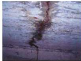
0220207-20111220-0015- Culvert~Longit crack at sof...
