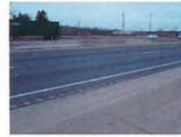
0220207-20111220-0002- Deck Surface~Surface alo...
