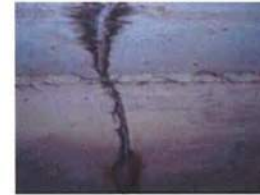
0220207-20111220-0012- Culvert~Longit crack w effl...
