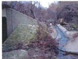
0220207-20111220-0024- Channel~Debris at N chan...
