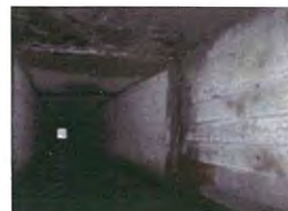
15 - Water seeping stalagmites and rust at cons...
