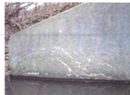
08 - Efflo and erosion behind WW typ
