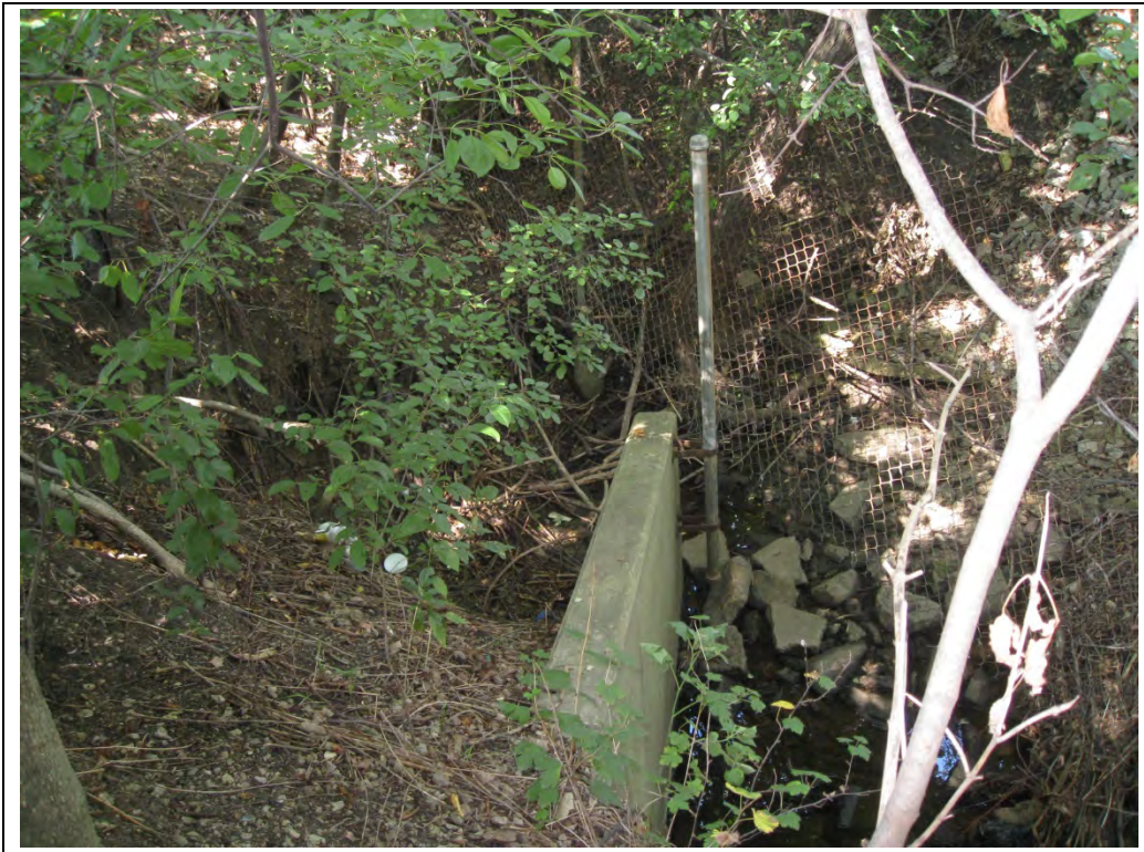
Photo #30 – Wards Creek Culvert – Erosion behind Northwest Wingwall (Looking North)
