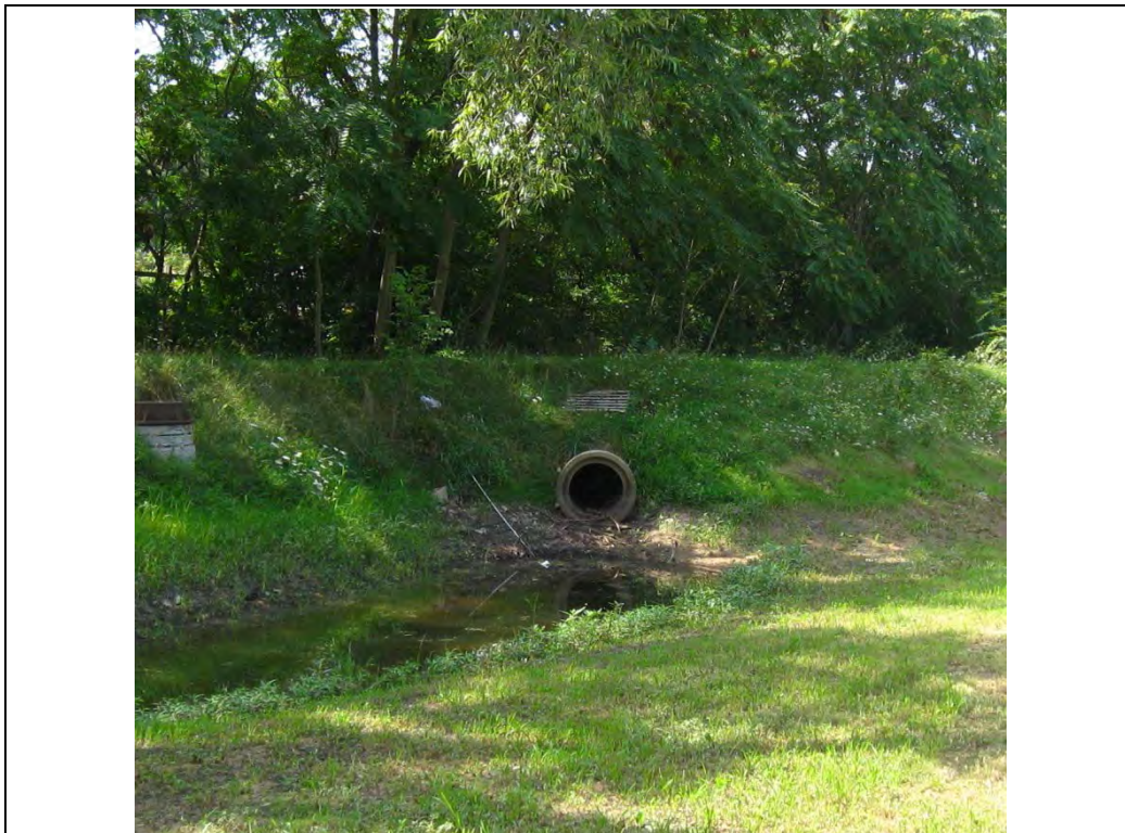
Photo #4 – Upstream End of 24” RCP Culvert through Golf Course Berm (Looking Southwest)
