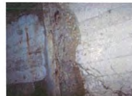
24 - Spall by construction joint at N section
