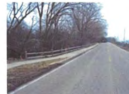
34 - Location N Frontage and pavement condition
