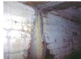
23 - Vert cracking w mineral deposit in walls typ S sec...
