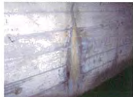
12 - Vert cracking w mineral deposit in walls typ S sec...
