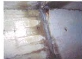
19 - 1 to 2 ft of delam rust seepage vert cracks and s...
