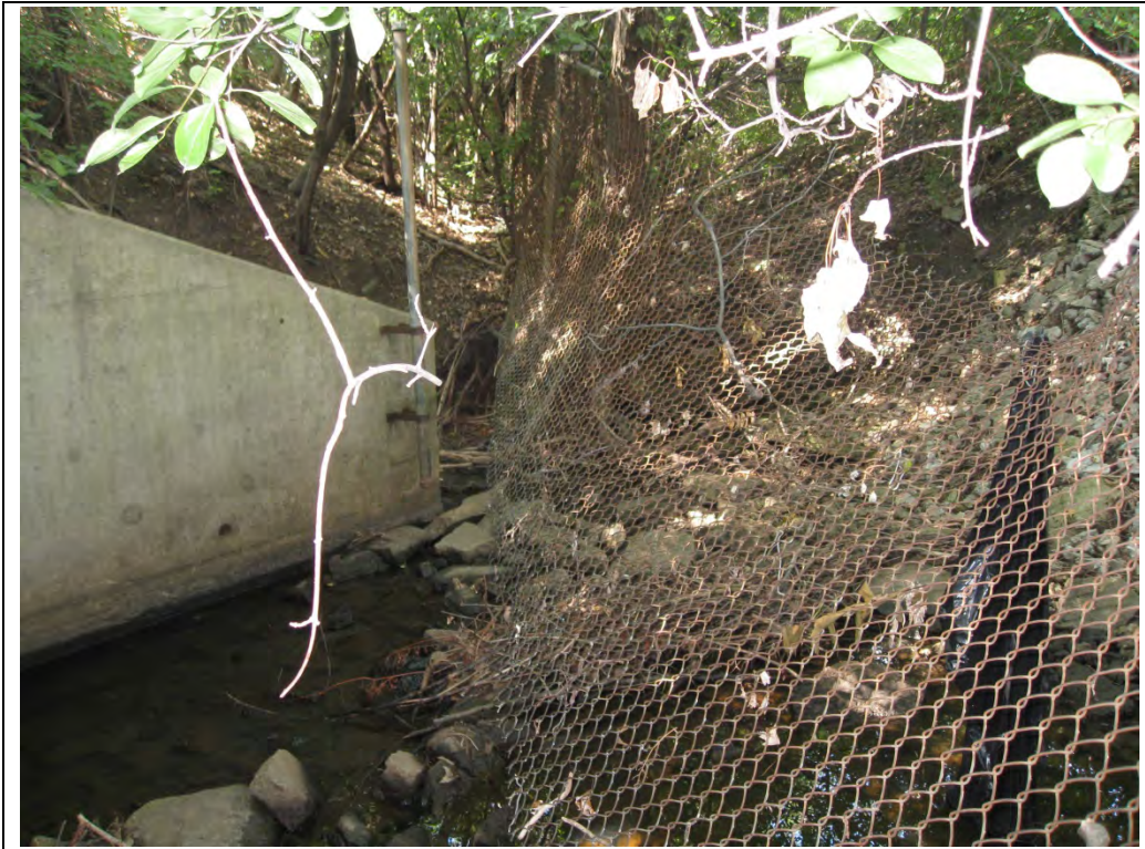
Photo #31 – – Wards Creek Northwest Wingwall – Erosion behind Northwest Wingwall (Looking West)
