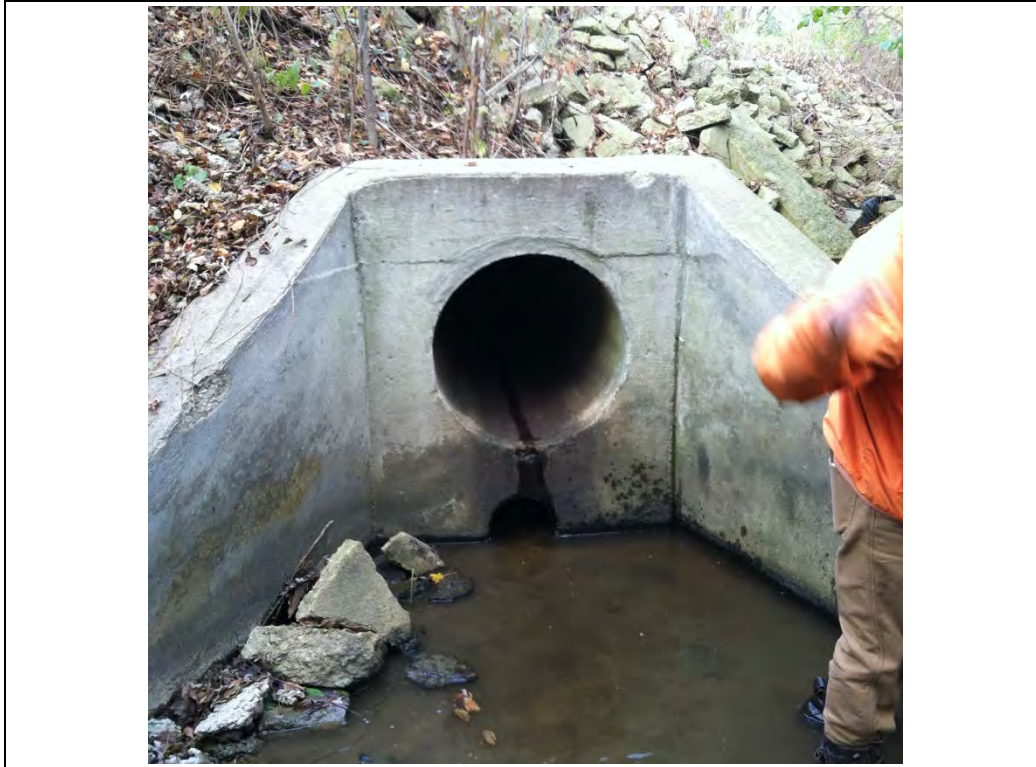
Photo #3 – Downstream Face of 10” & 24” RCP Culvert through Golf Course Berm (Looking Northeast)
