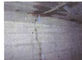
29 - HL cracking at walls and top slab Mineral deposit r...
