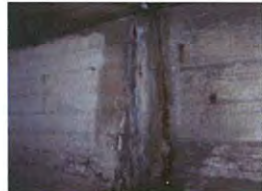
16 - 1 to 2 ft of delam rust seepage vert cracks and s...
