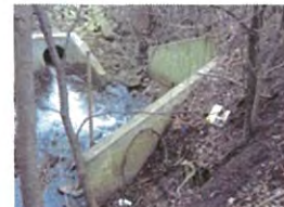
33 - Important erosion behind NW WW THREA...
