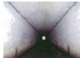
20 - General condition at N section
