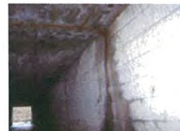
30 - Vert cracking rust seepage and delam by co...
