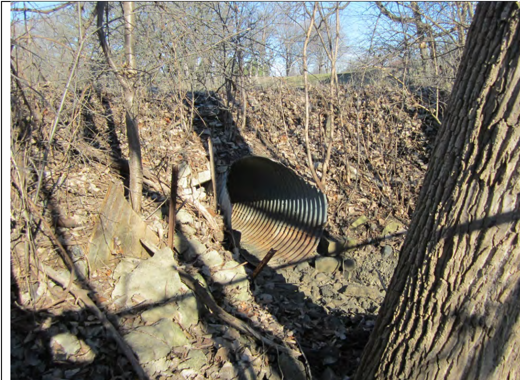
Photo #6 – Downstream Face of 30” CMP Culvert through Golf Course Berm (Looking East)
