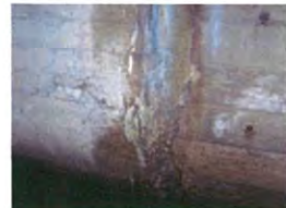
18 - 1 to 2 ft of delam rust seepage vert cracks and s...
