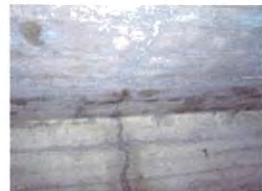
13 - HL cracking at walls and top slab Mineral deposit r...
