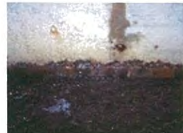
27 - Possible scour and water seepage along interf...
