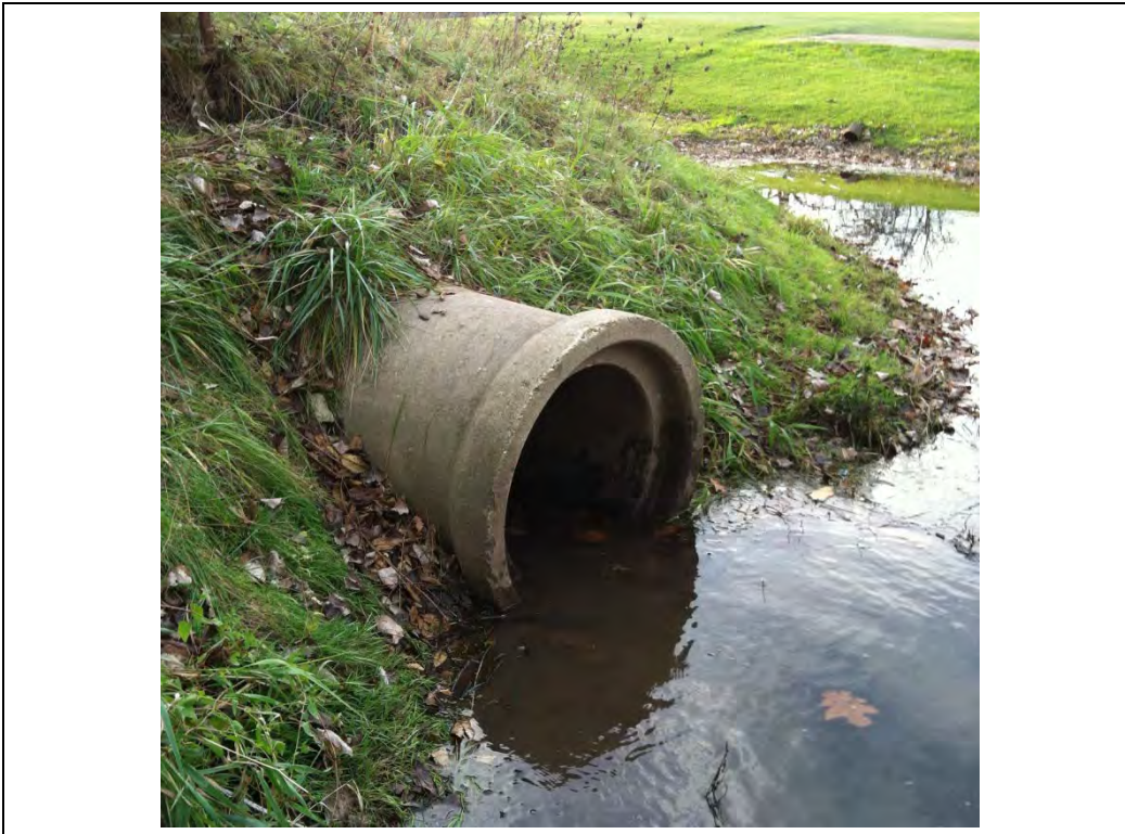
Photo #5 – Upstream End of 24” RCP Culvert through Golf Course Berm (Looking West)
