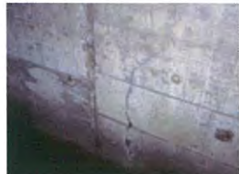
11 - Scattered lower half vert cracking in walls worse at...
