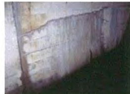
22 - W wall N section horiz crack w chloride vert crac...
