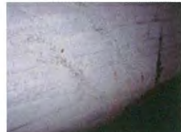
26 - Low concrete and vibration quality
