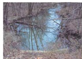
04 - Downstream S Channel Note moderate erosion
