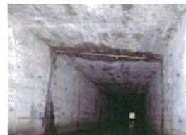
14 - Water seeping at construction joint Stalagti...
