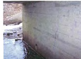
31 - HL vert cracking at N end
