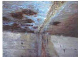
17 - Spalls and rust spots at const joints at S to mid sec...
