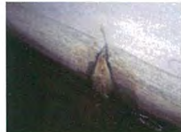
21 - Bottom wall vert cracking and mineral depo...
