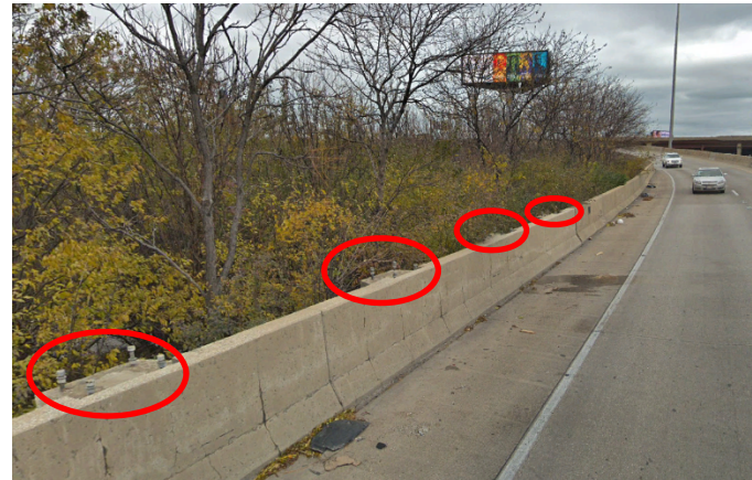
Southbound I-90/I-94 to Southbound I-55 Ramp, facing northeast Structural supports circled in red
