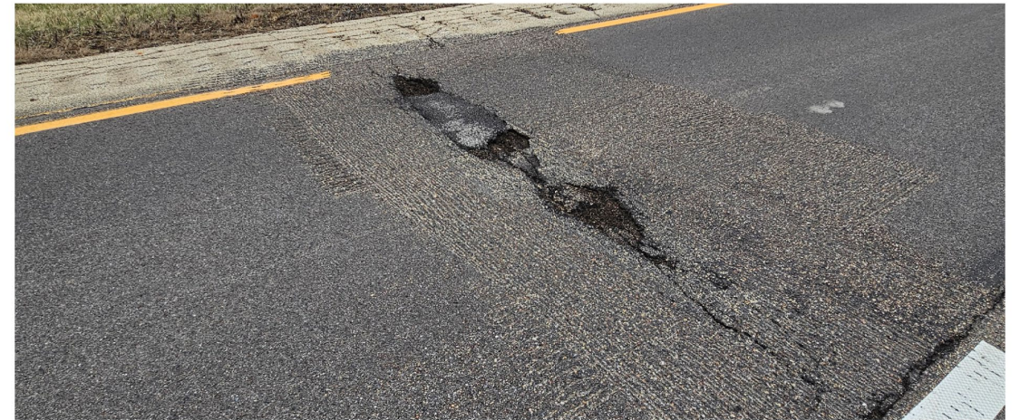
(Pavement conditions along the project study area on US 20)
