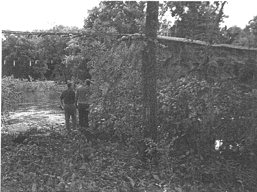
Chicago Northwestern Railroad Embankment Failure
