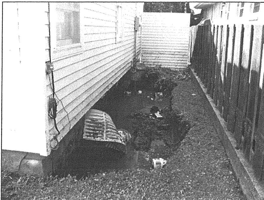
Basement collapse from the force of the flood waters. Photo from NWS web site
