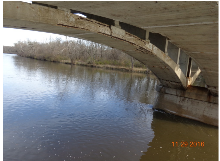
Arch Deterioration (Span 2)
