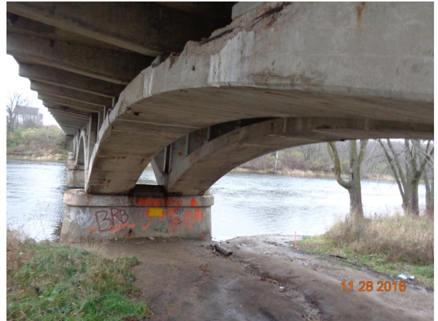
Arch Deterioration (Span 5)
