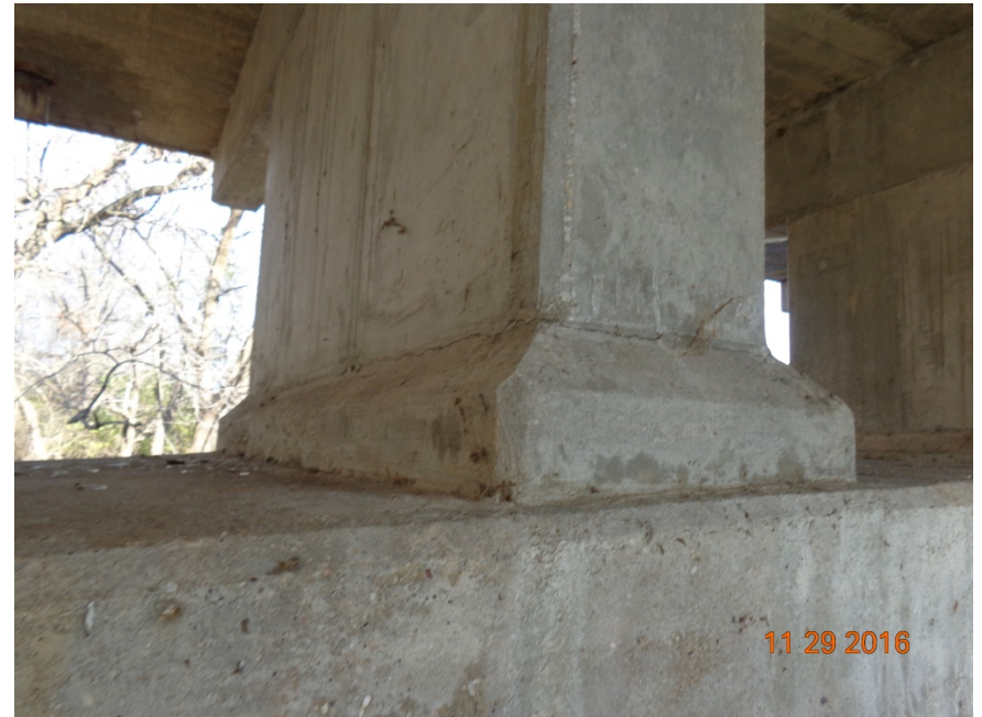
Crack in Column at Base
