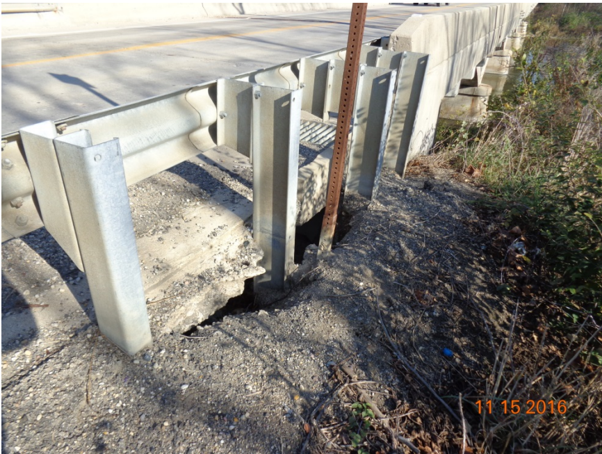
Void under South Side of West Approach Shoulder
