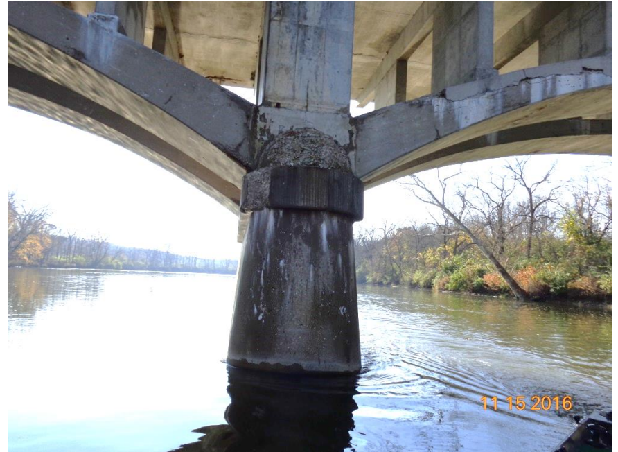
Typical Pier Nose Deterioration
