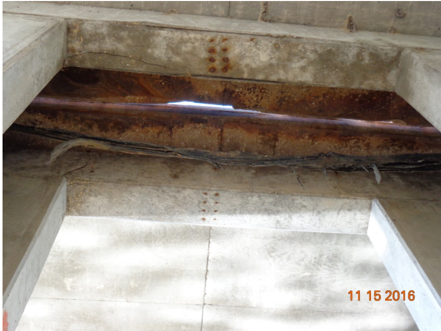
Deterioration Under Joint
