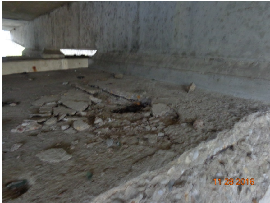
Top of Arch Delamination & Spall
