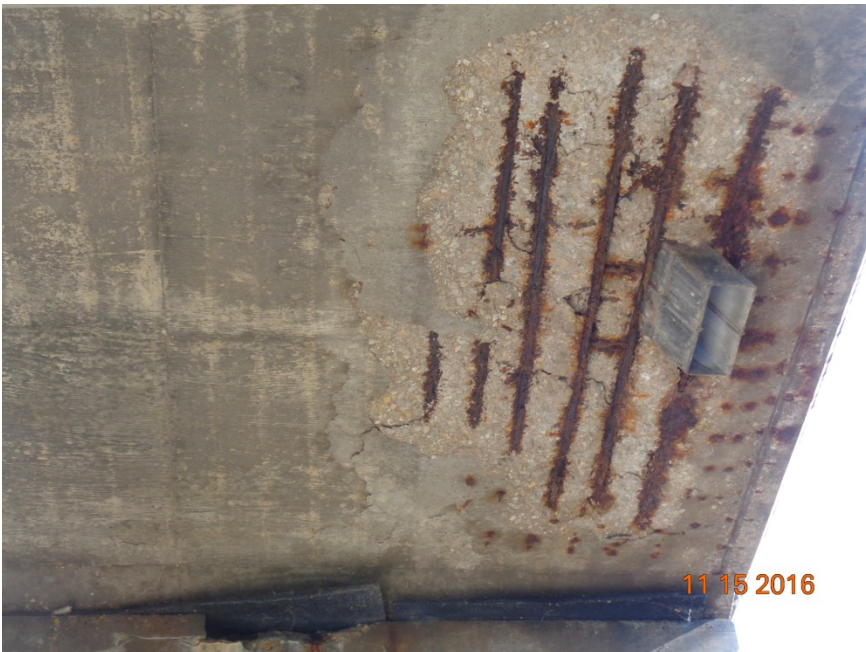
Spall at Deck Drain and Bearing Pad Movement at East Abutment
