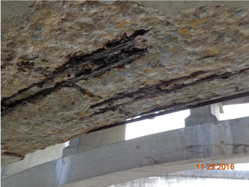
Spall on Underside of Arch
