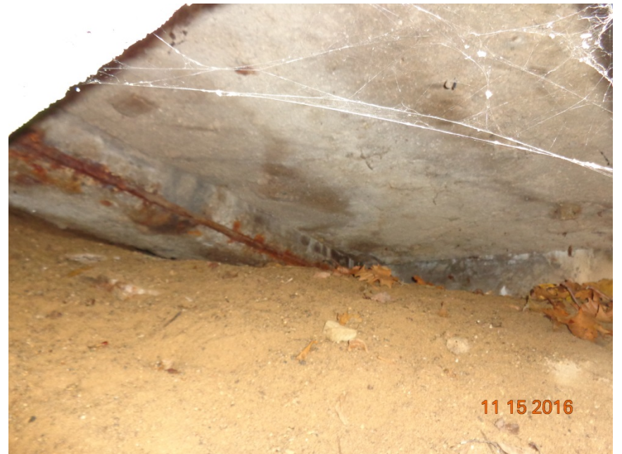
Void Under West Approach Slab
