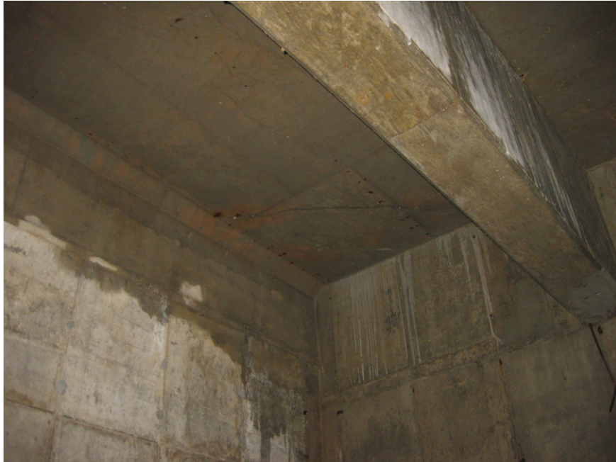
Typical Crack in Deck and Leakage inside Vaulted Abutment
