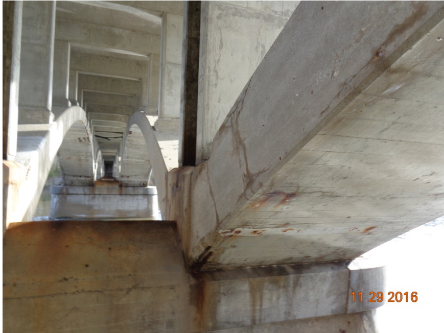
Hairline Cracks in Arch near Pier 1
