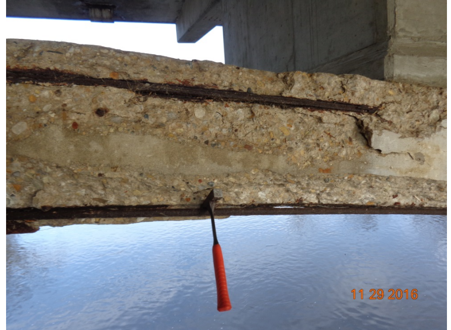
Debonded Arch Reinforcement
