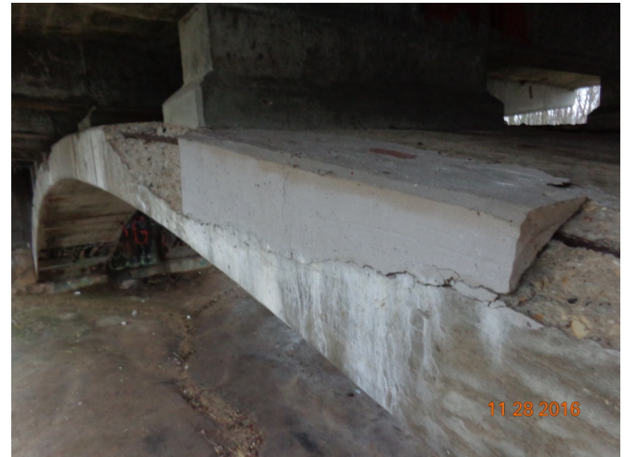
Failed Patch on Arch
