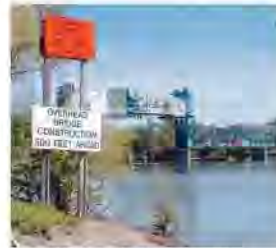
Work continues to prepare construction plans and specifications to repair the Illinois River lift bridge, which closed in June because of structural issues discovered during a routine inspection. (H-W File Photo)
