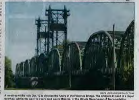
A meeting will be held Oct. 12 to discuss the future of the Florence Bridge. The bridge is in need of a major overhaul within the next 10 years said Laura Mlacnik, of the Illinois Department of Transportation.
