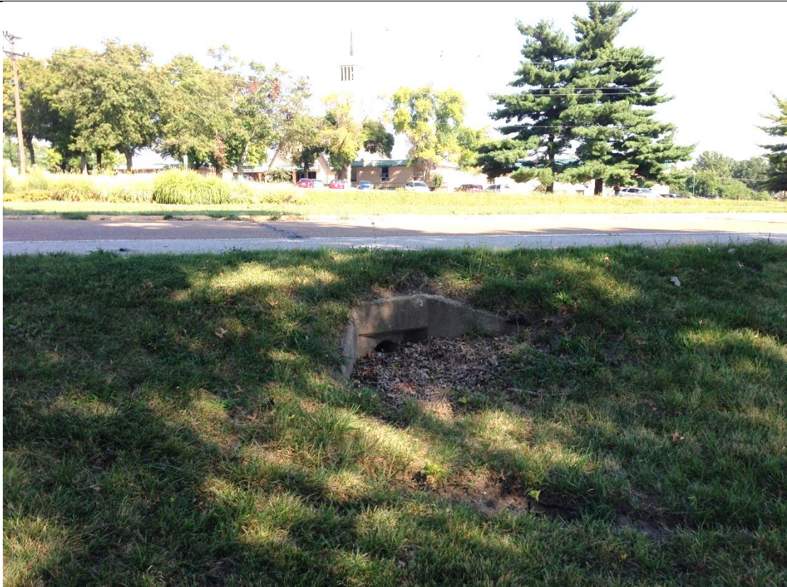
Cross Road culvert (18" RCP) under IL 3/ W. Homer Adams Pkwy looking north
