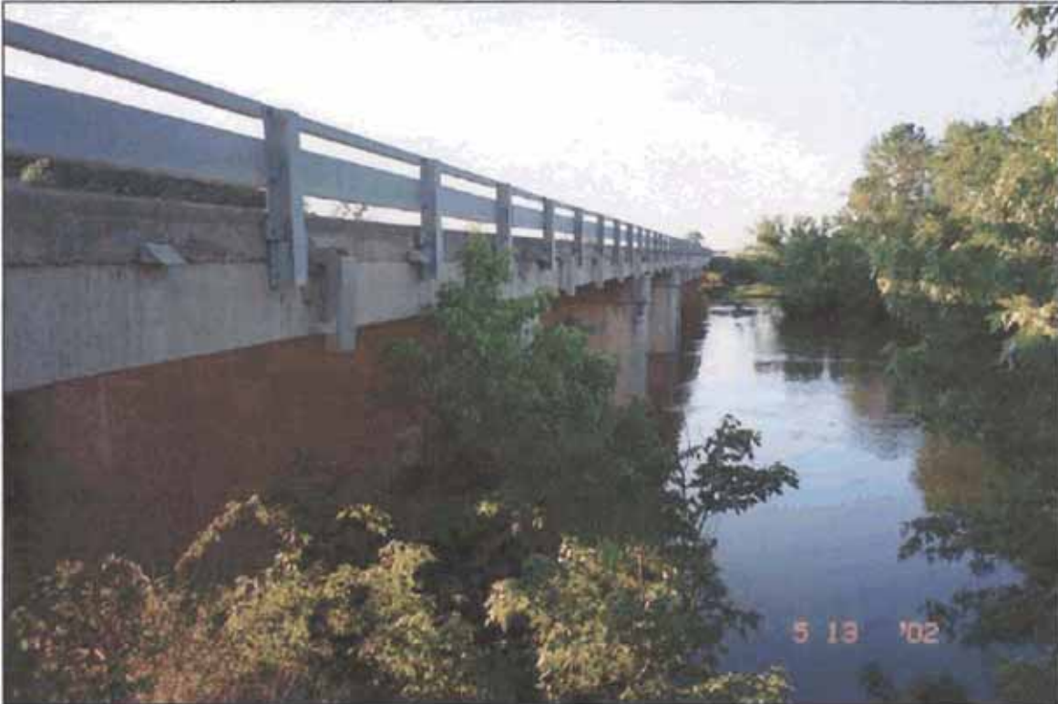
DOWNSTREAM (EAST SIDE) FLOODED CONDITION
