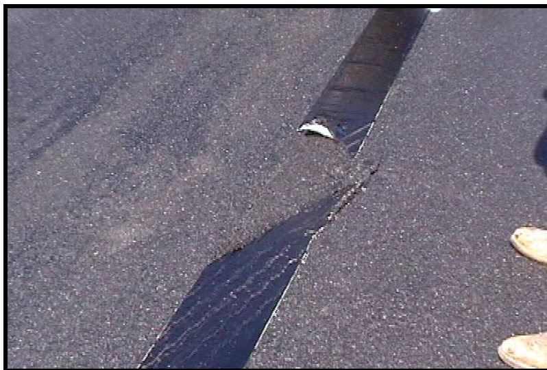
Figure 46: Joint Sealant Tracking
