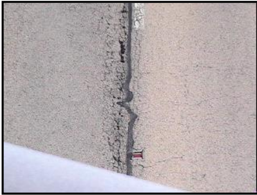
Figure 4: Joint Distress with Sealed Joint
