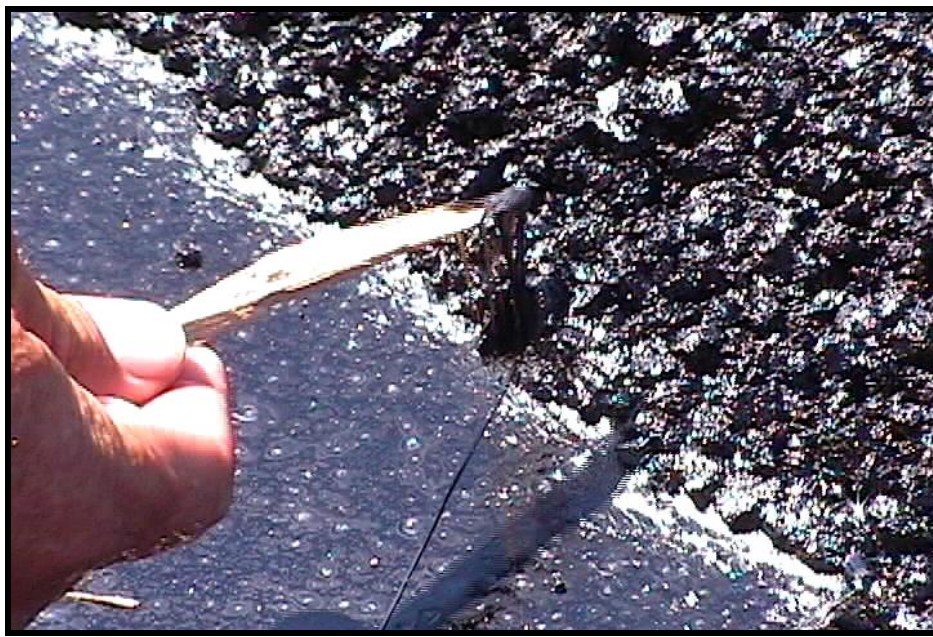
Figure 47: Joint Sealant Softens under HMA Surface
