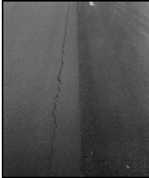
Figure 10 J-Band® Boundary Cracking
