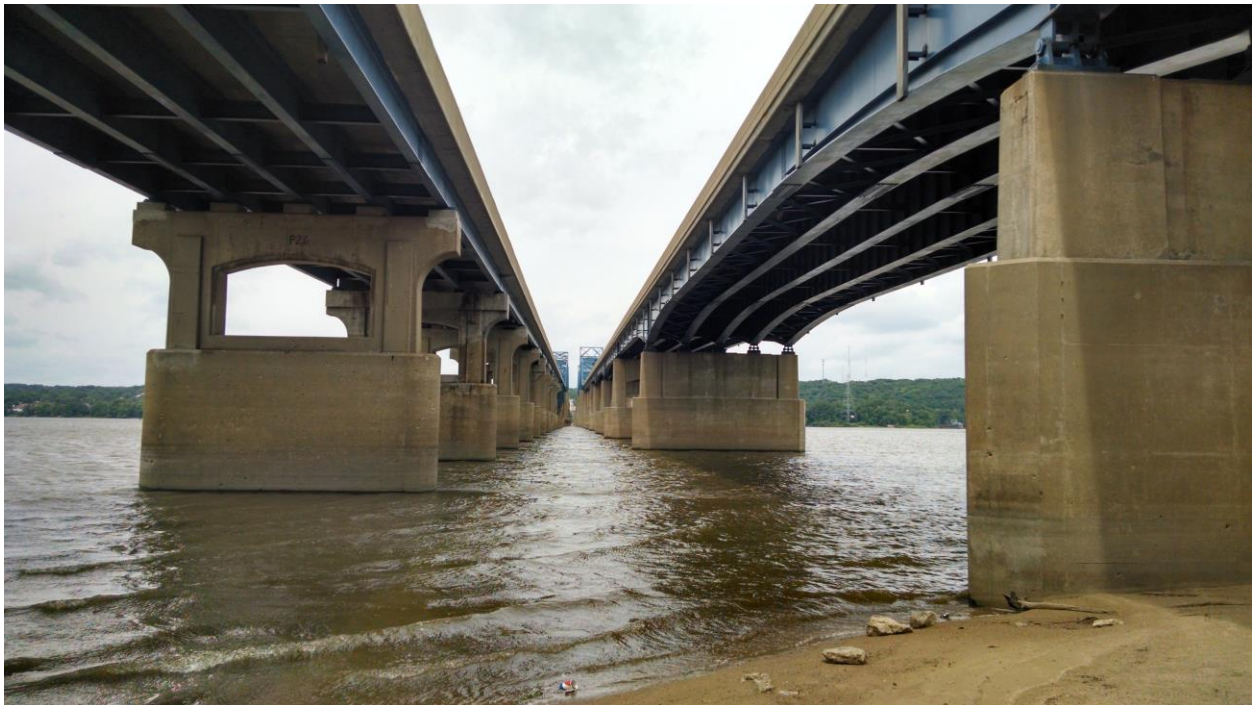
At east shore of the Illinois River under US 150 (eastbound bridge on left) facing west
