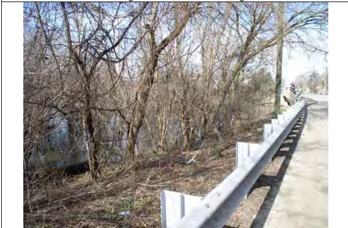
Photo 04 – FPDCC Big Bend Lake Woods located south of Rand Road. Looking West to Rand Road Bridge.
